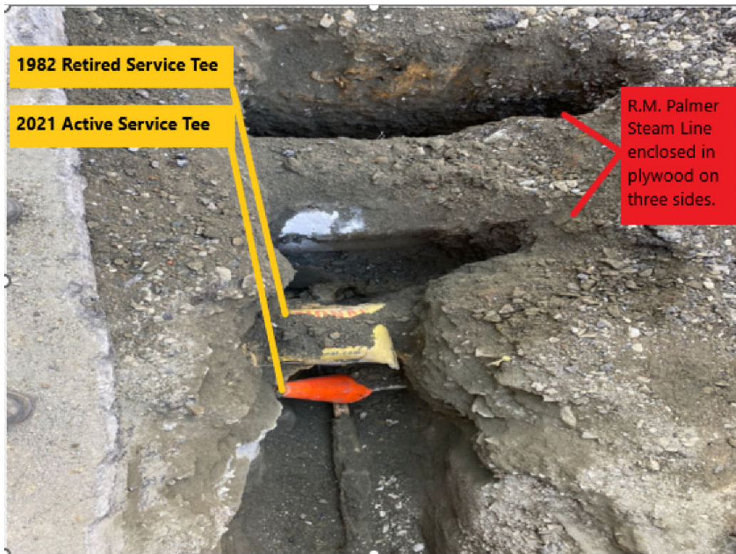
Figure 1: April 24, 2023, Excavation of R.M. Palmer Steam Line, facing West (Courtesy of PA PUC Image 2393)
