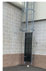
Locked Roof Access Ladder
