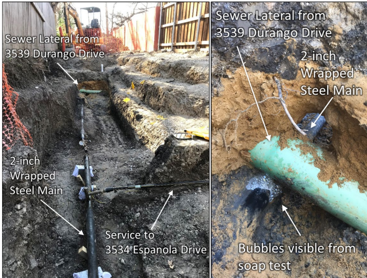
Figure 7. Crack in natural gas main at 3539 Durango Drive sewer lateral crossing. (Courtesy of Atmos.)
