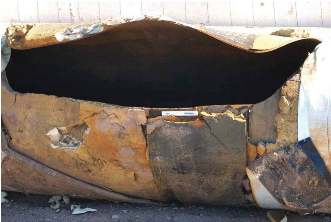
Photograph 1. Representative documentation of the hydrotest rupture at MP 493.1.
