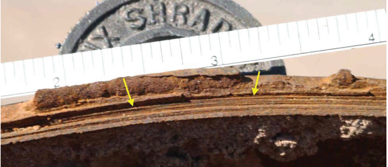
Photograph 3. Another portion of the hydrotest rupture surface at MP 487.5 showing more of the part-wall defect (arrows).
