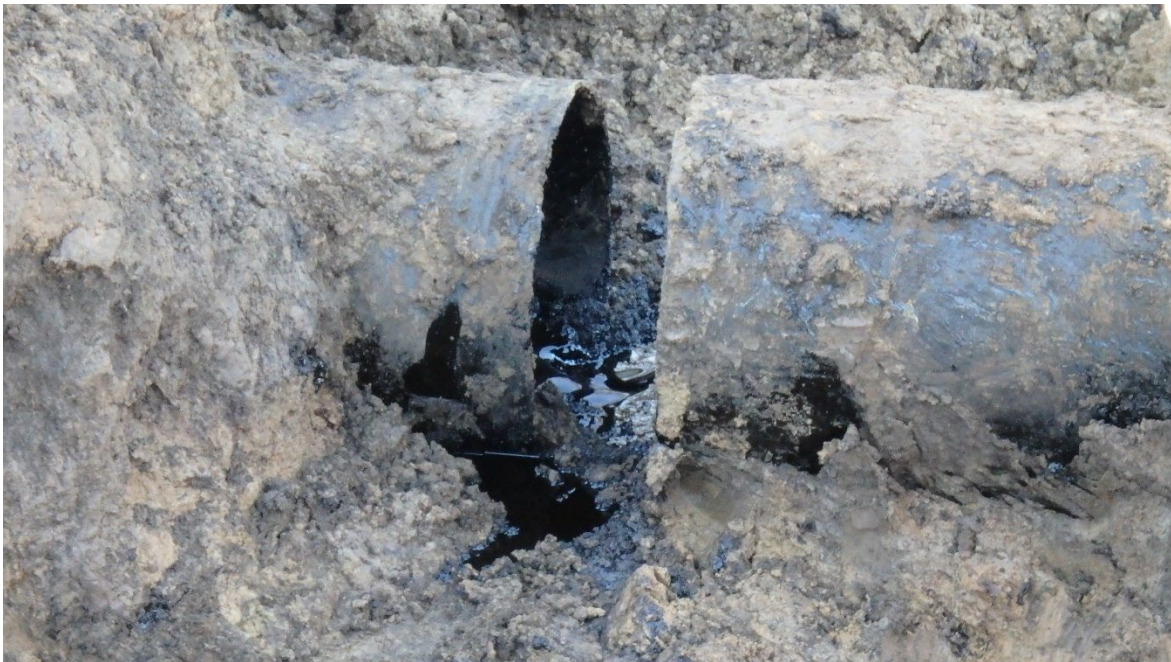
Figure 6. Close up of the Woodpat pipeline separated at the girth weld. (March 12, 2022, 7:00 p.m.)
