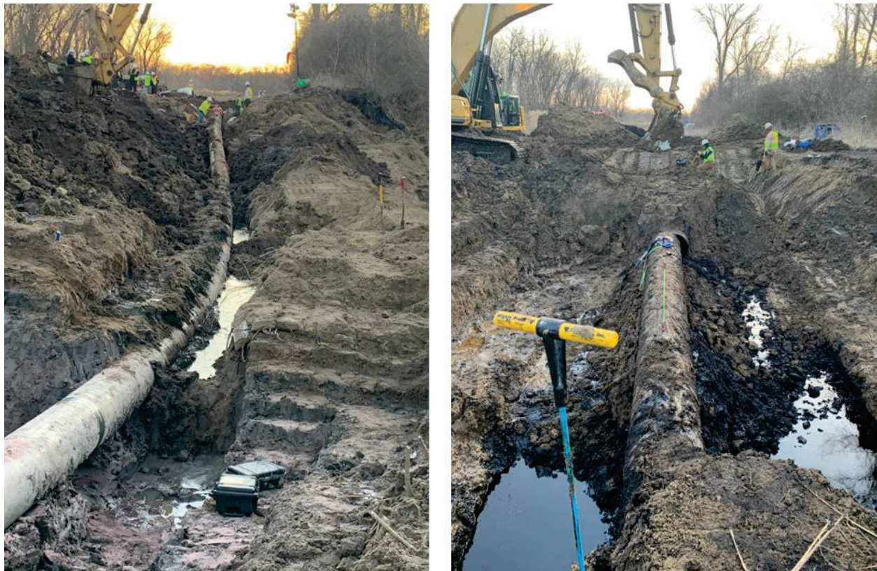
Figure 1.1: Failed Girth Weld During Excavation
