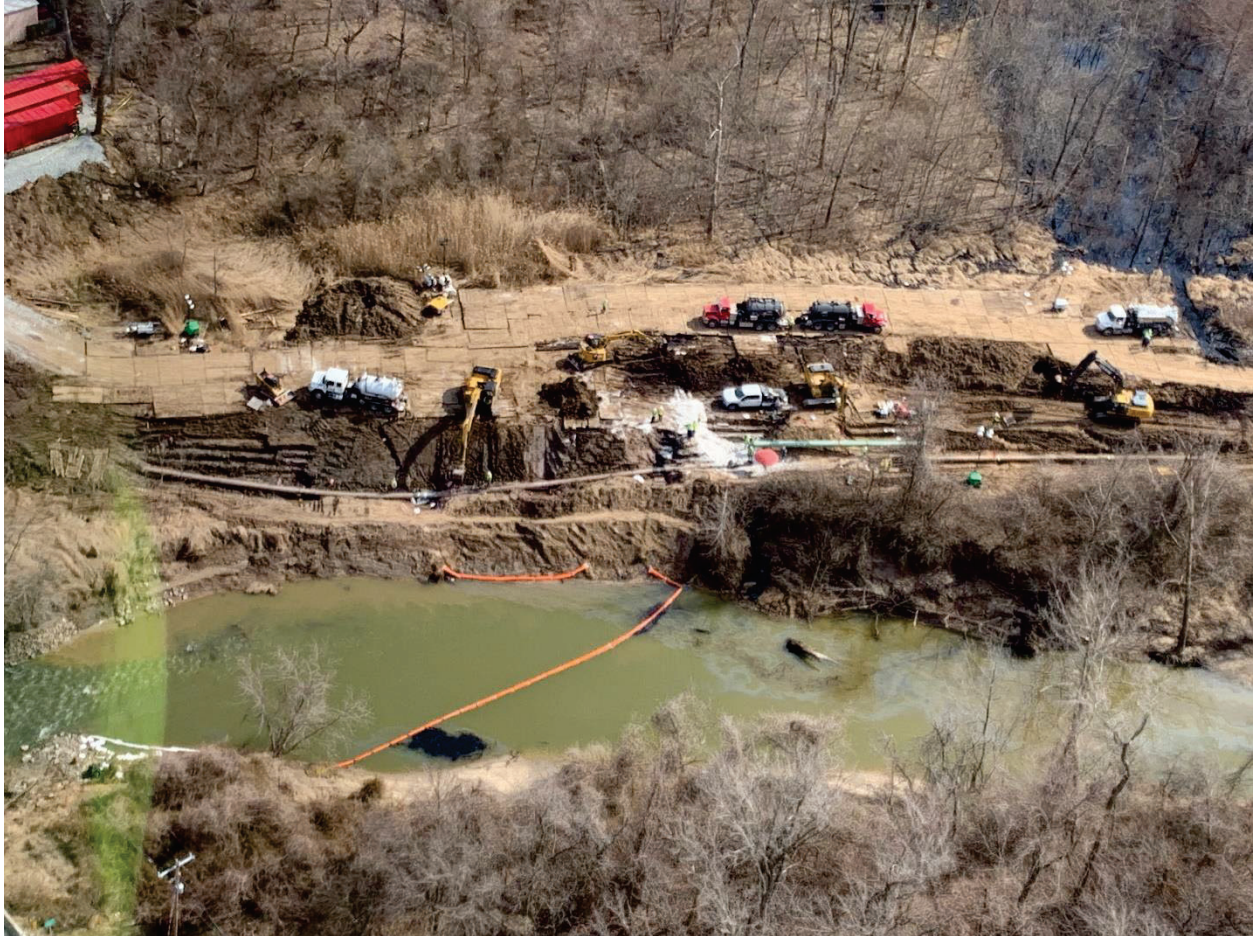
Figure 1.2: Aerial Image of Failure Location
