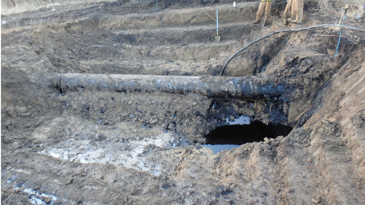
Figure 5. Woodpat pipeline point of failure. (March 12, 2022, 7:26 p.m.)
