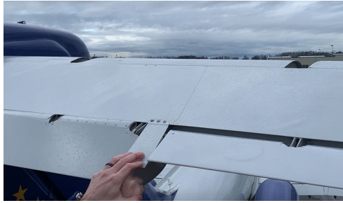
Figure 5. Elevator as viewed in trailing edge down from an elevated position aft of the aircraft looking forward, with manual downward pressure being applied during control column aft movement.
