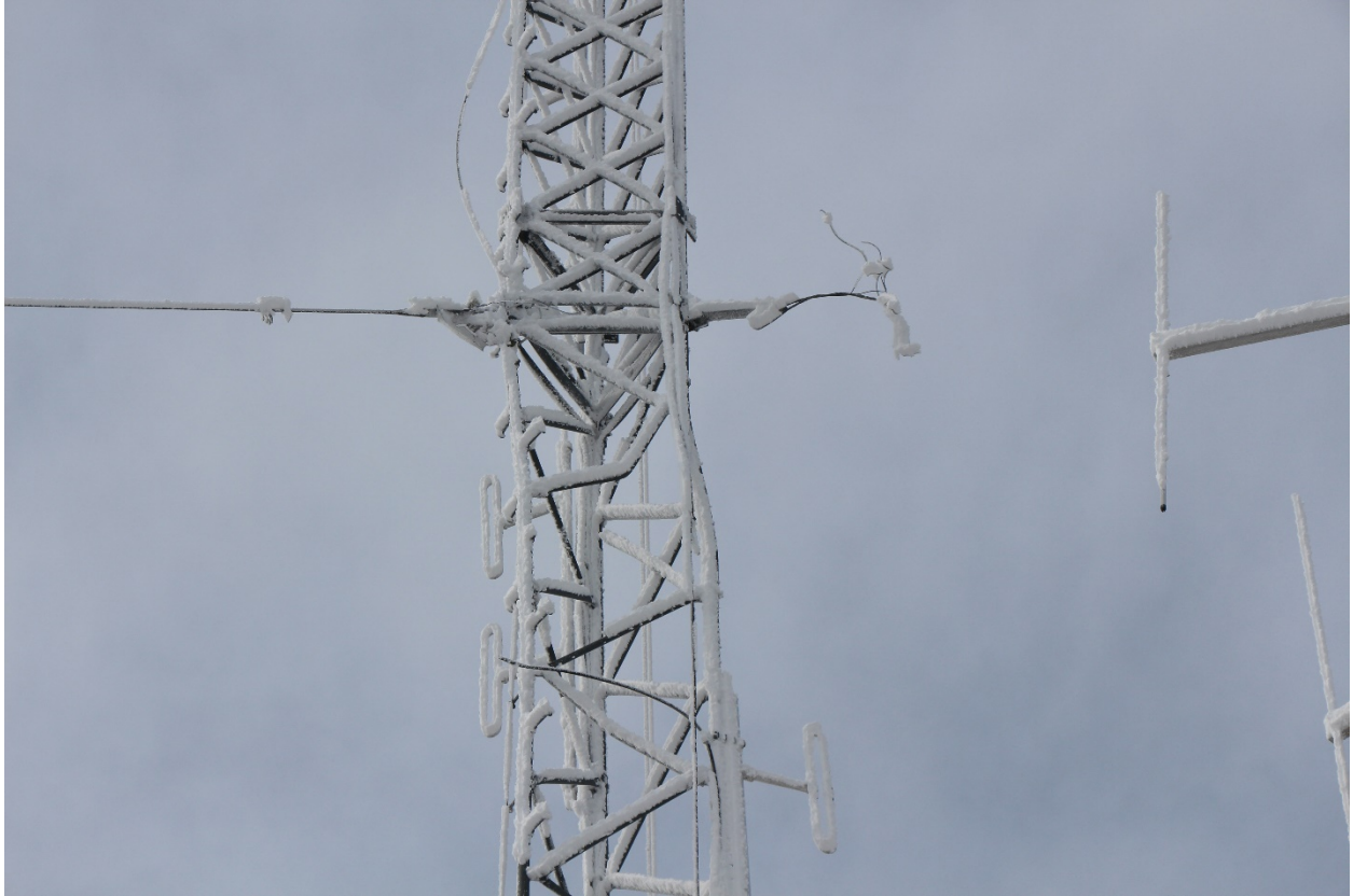
Photograph 2: Radio Tower Damage
