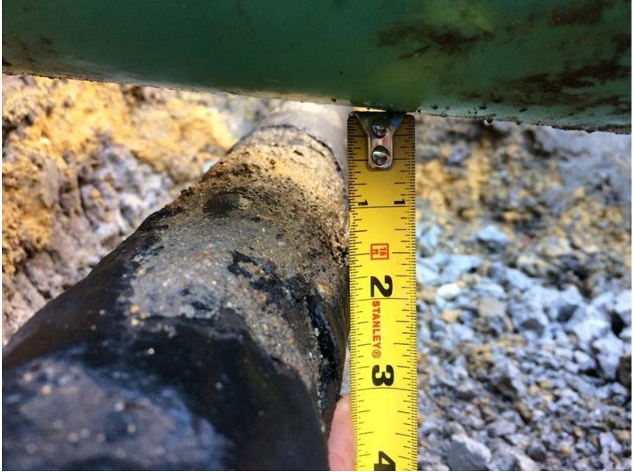
Figure 5 — Separation of 1.5" between the damaged top of the Main and the bottom of the sewer lateral.
