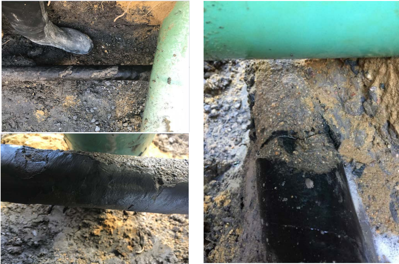
Figure 4—Damaged section of the Main relative to the sewer lateral serving 3539 Durango and the circumferential crack.
