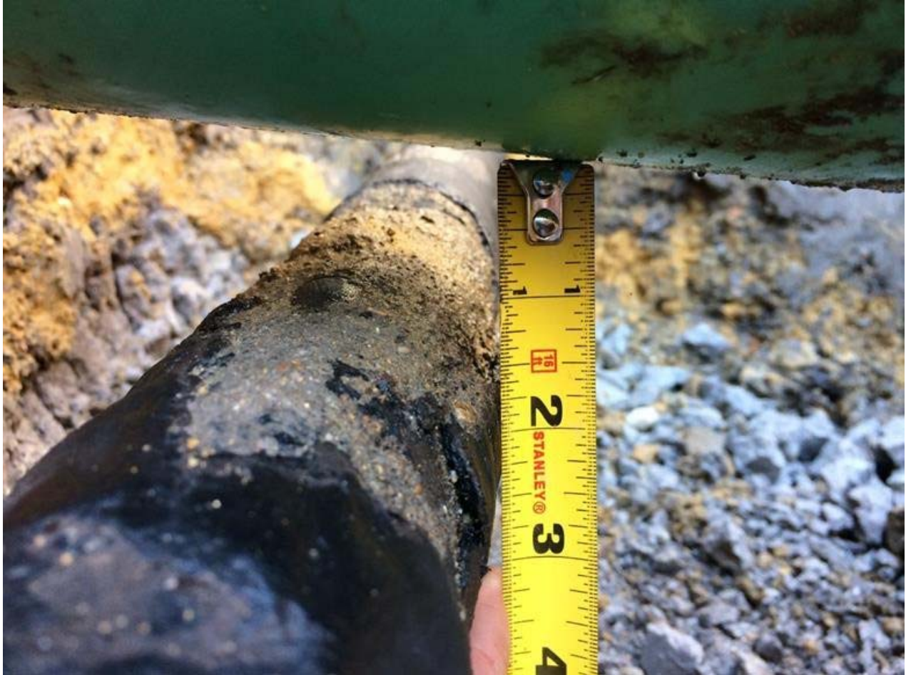
Figure 5 — Separation of 1.5” between the damaged top of the gas main and the bottom of the sewer lateral.
