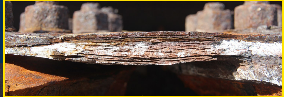
Lamellar corrosion in connecting plates
