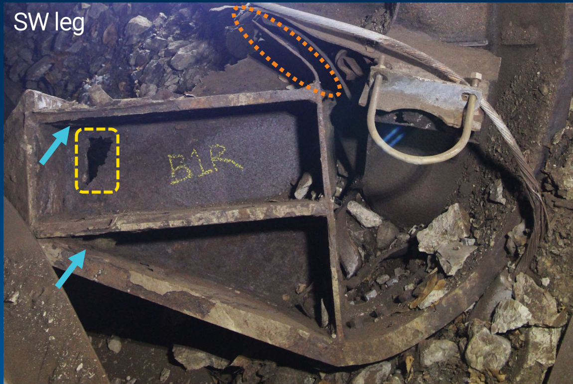
Corrosion product build-up
