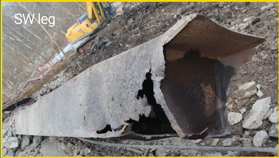
Holes in cross-bracing end
