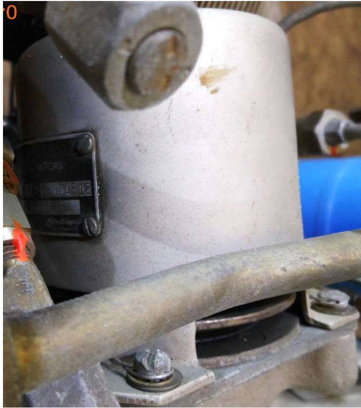
Photo #6 – Pressure Relief Valve
