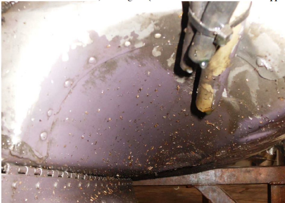
Photo # 2 – Left exhaust tunnel, looking aft (breather and drain tubes seen upper right)
