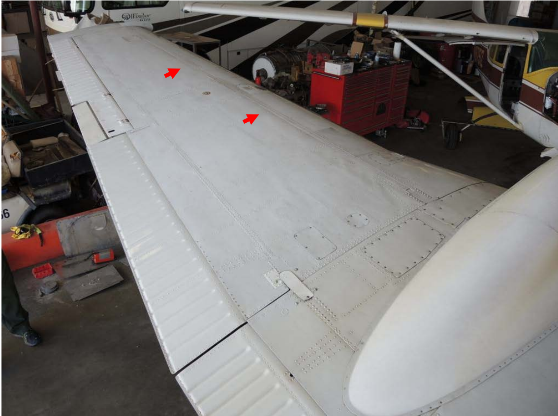
Figure 12. Wrinkles in the top skin of the left wing, immediately outboard of the engine and aft of the forward spar. The arrows indicate skin raised as a ridge aft of the outboard section of the forward wing spar. (Also visible in photos from the delivery flight to Hawaii in Figure 18) (Photo from: Textron Report ASI-16-CF, taken August 11, 2016)
