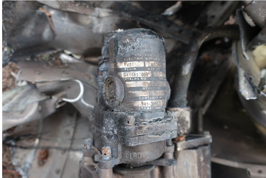
Figure 59. Fuel shutoff valve found in open position. (Photo from: Swaim)
