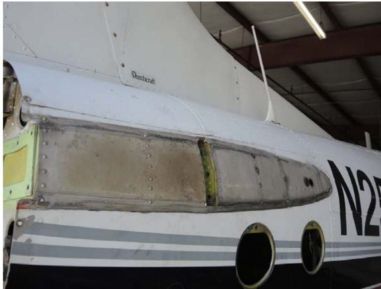
Figure 5. The right rear fuselage with a bend in the bulkhead which the right HSTAB attached to. (Photo from: Textron Report ASI-16-CF, taken August 11, 2016)
