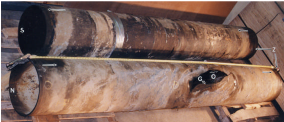
Figure 1. Pipe section showing the location of the gaping crack (G) and crack origin (O) after removal from the field. North and south ends are indicated by “N” and “S”, respectively. Pipe was cut in the field in the area indicated by arrows “Z”.
