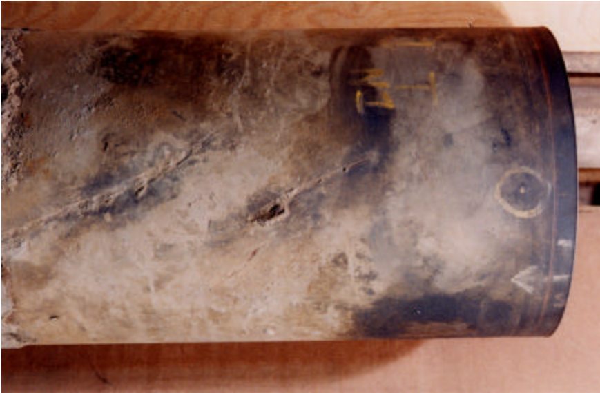
Figure 2. Close-up photograph (left) of the north end of the pipe showing two exposed diagonal gouge marks. Specimen labeled “E” was removed from the gouge mark located at the upper left corner of the photograph.
