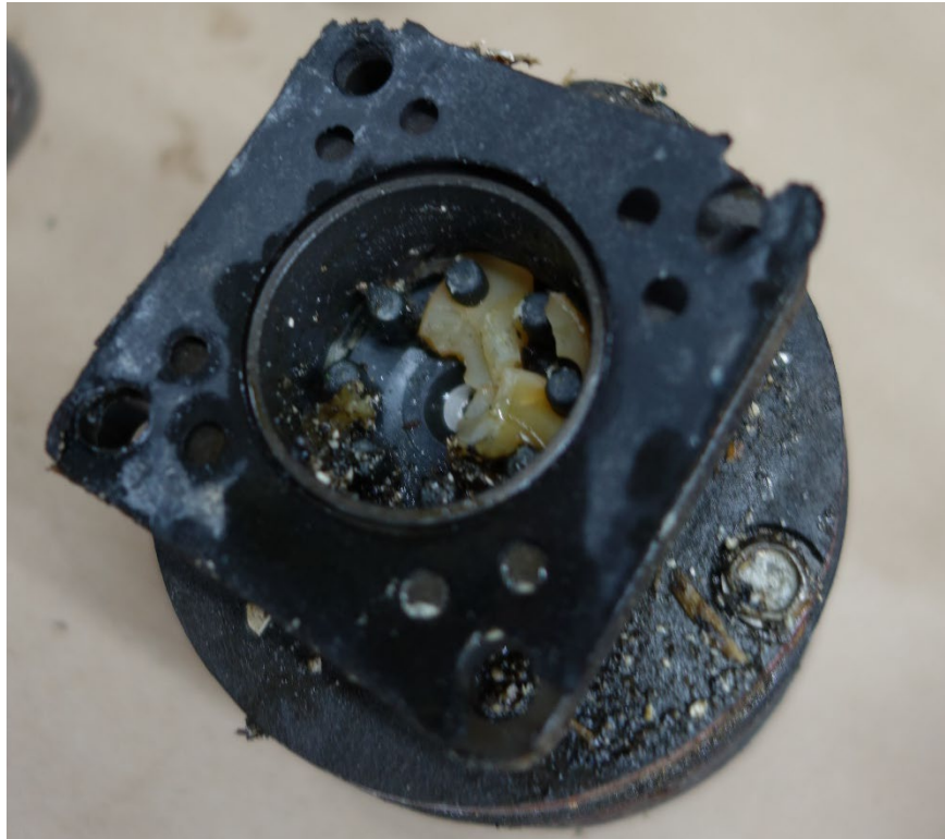
Photograph 4 – Vacuum pump - partial drive coupling.
