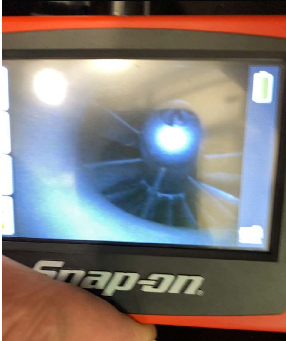
Figure 4: Photograph of the unobstructed engine air inlet.
