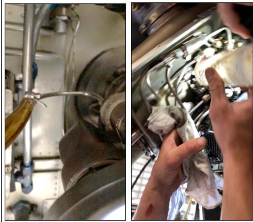
Figure 2: Photographs taken during the PC line pressure check, while fluid was applied to the lines
