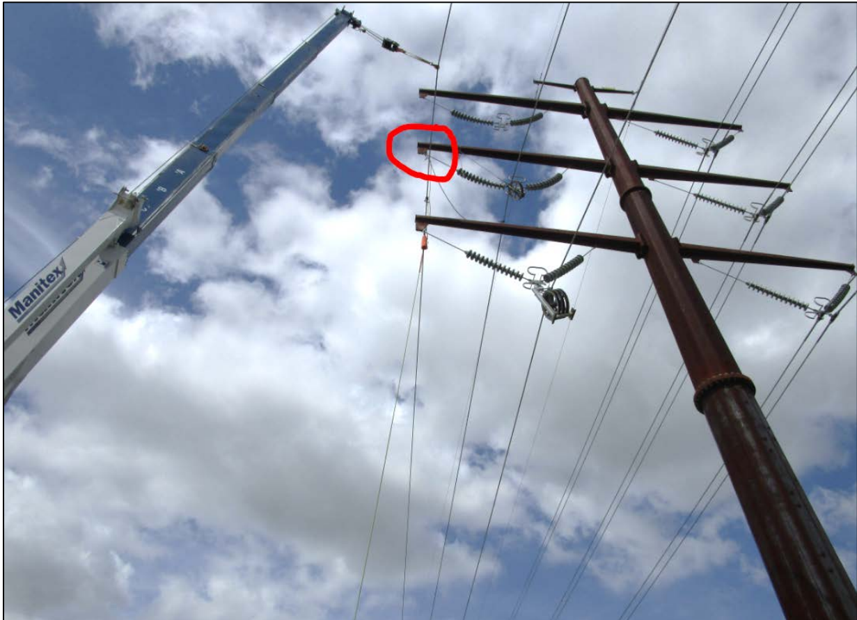
Figure 1: View of the conductor powerline that was moved by the helicopter
