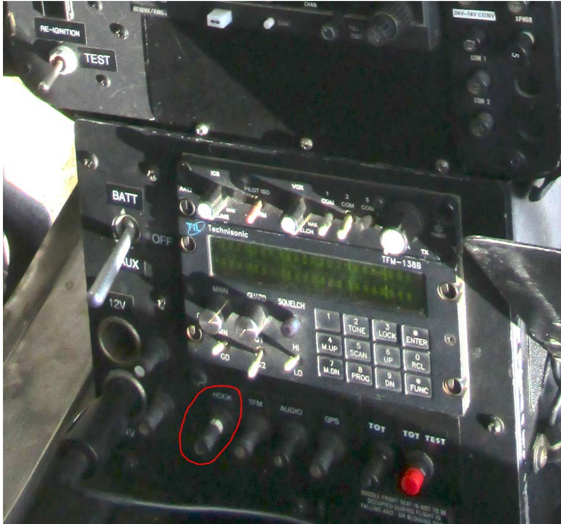
Figure 6: View of the pulled circuit breaker that controls the hook release button located on the cyclic
