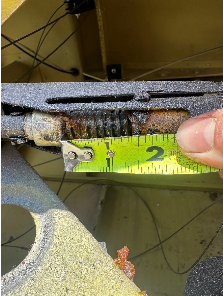
Figure 1: AAR Digital Photograph. View of Measurement of the Rudder Trim Control Tube Assembly Showing Being Extended 1.375 inches or About 8 threads.
