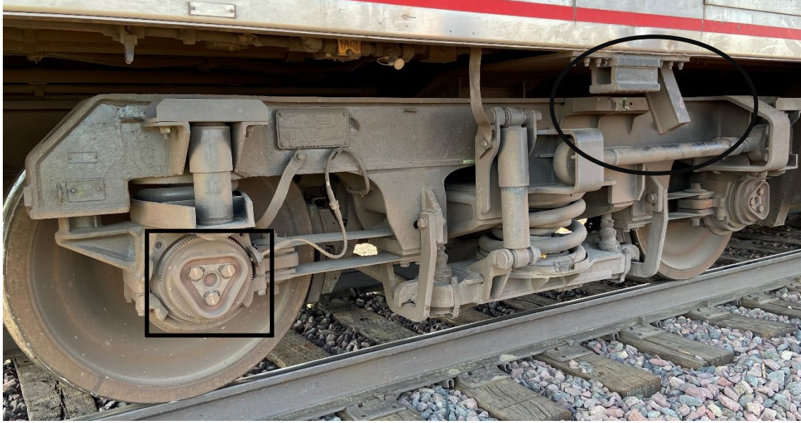
Figure 7. Photograph of the same 32050 truck with bump stop damage, taken by a different Volpe investigator.
