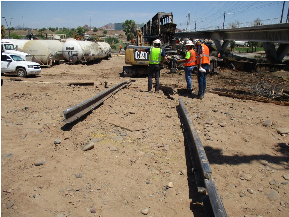
Figure 1 Photo of the accident scene at the south end of the bridge looking north. (Photo by FRA)
