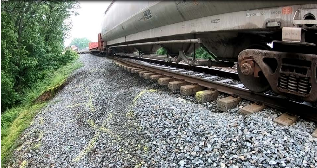
Figure 2. Failed roadbed at MP 102.85
