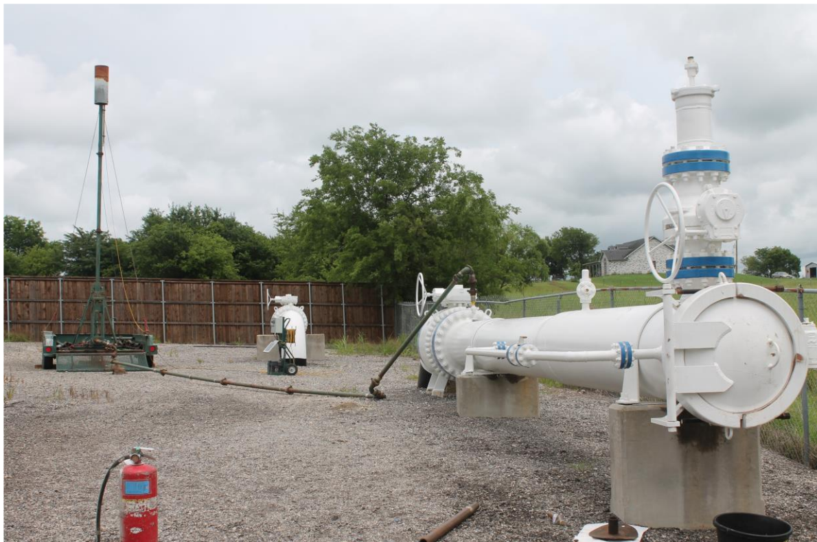
Figure 2: Launcher #2 connected to flare rig.
