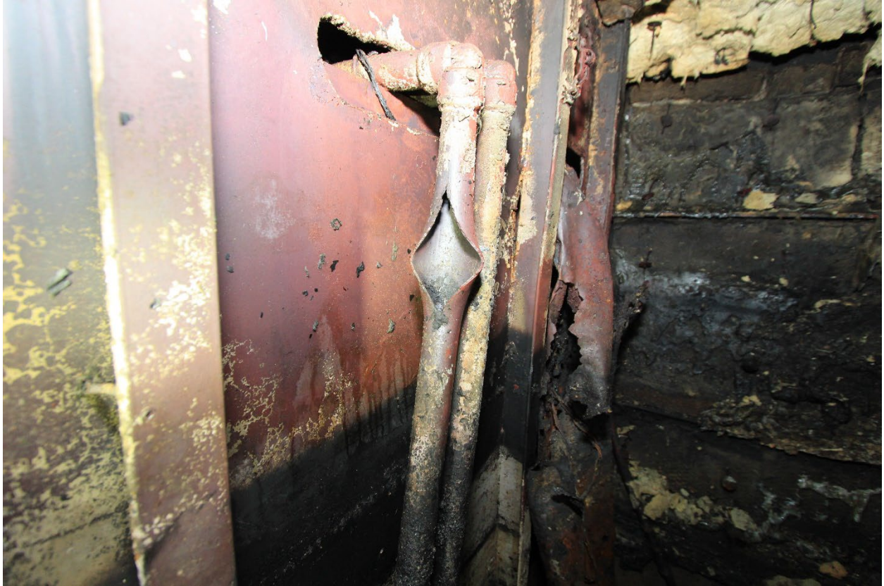
Figure 30. Hydraulic pipe fracture at ceiling near hydraulic power unit.
