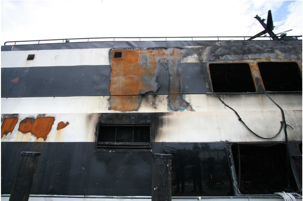
Figure 3. Starboard side engine room vent outlet.
