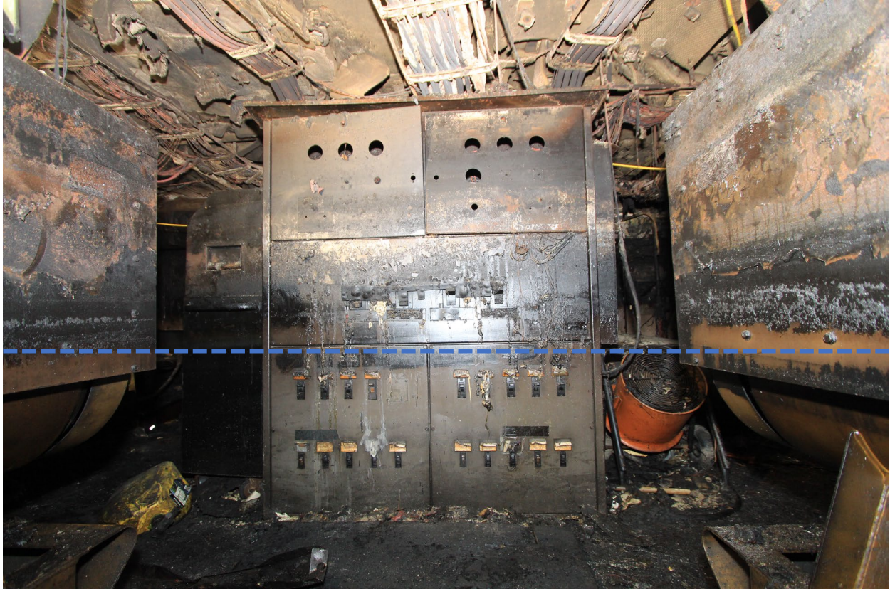
Figure 17. Electrical Cabinet with demarcation line.
