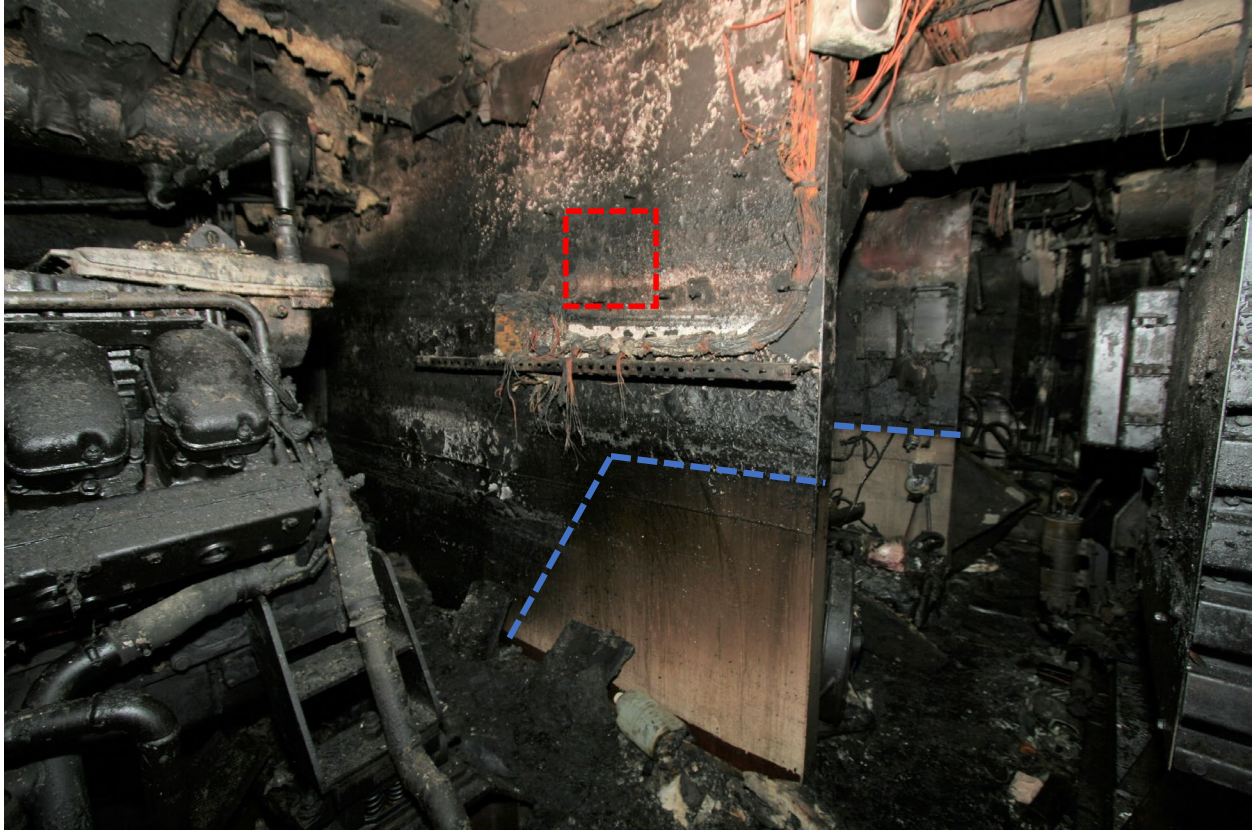
Figure 21. Bulkhead forward of port main engine with low lying damage towards the outboard side. Demarcation line shown (blue) and location of throttle controller (Red).
