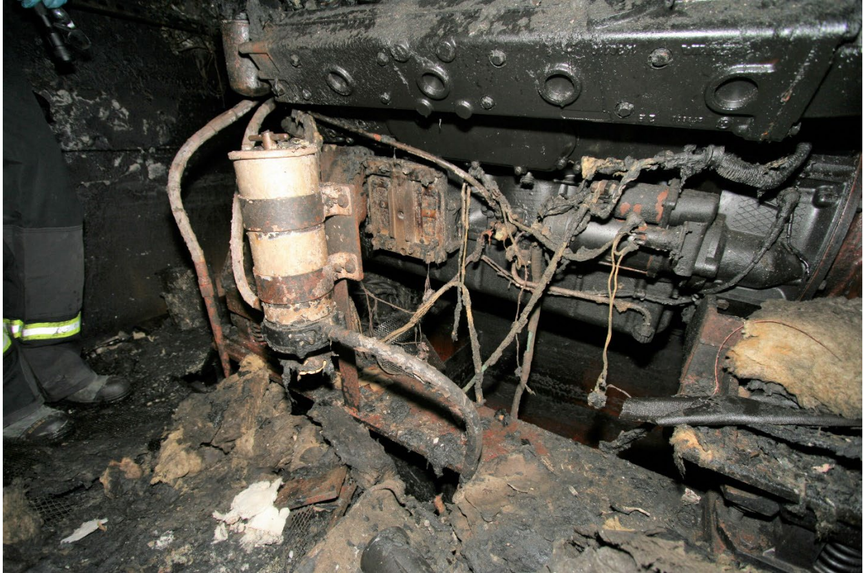
Figure 25. Outboard side of port main engine. Consumed fuel/water strainer bowl and low-lying charring to the deck level and below.
