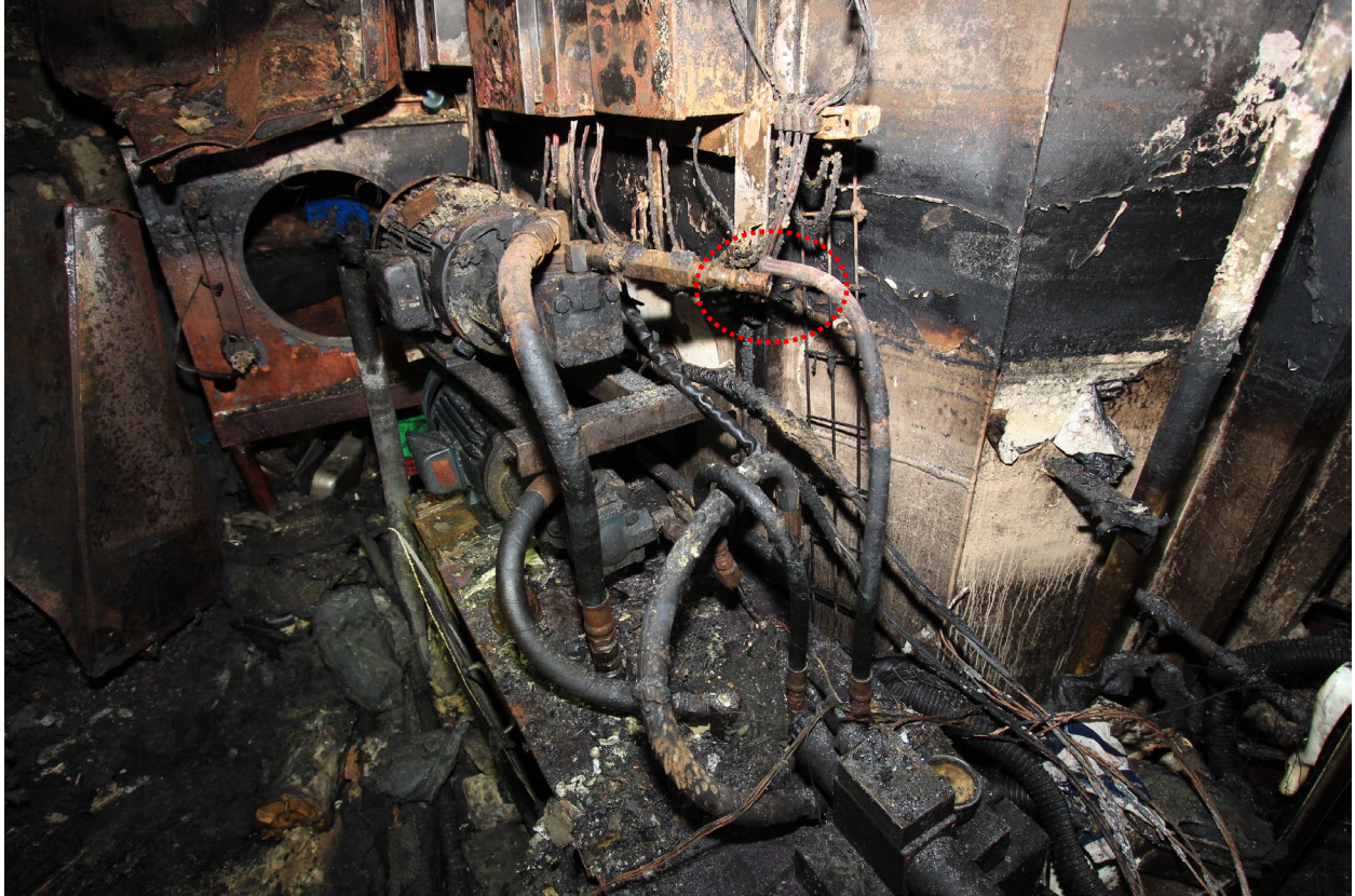
Figure 28. Hydraulic hose failure at pump outlet.
