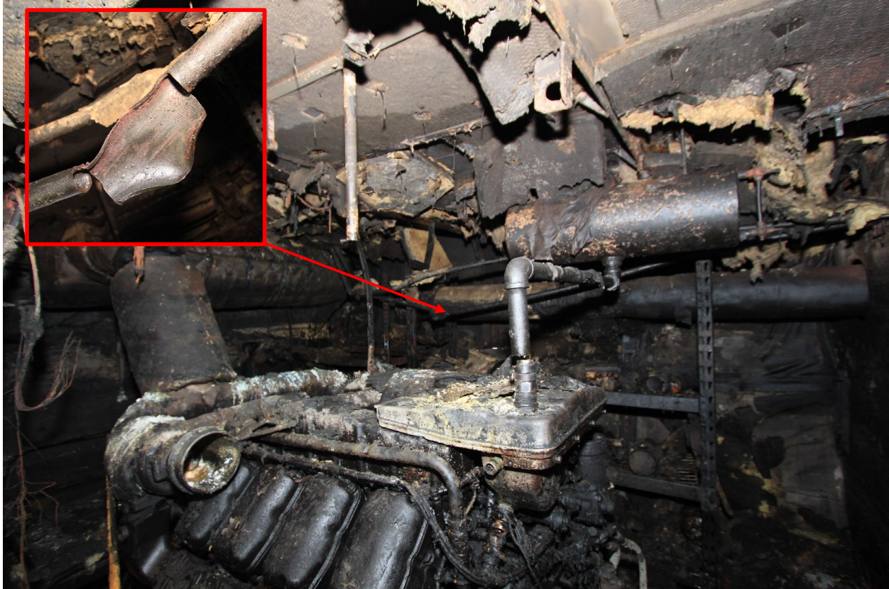
Figure 29. Hydraulic pipe fracture at ceiling height near port main engine.
