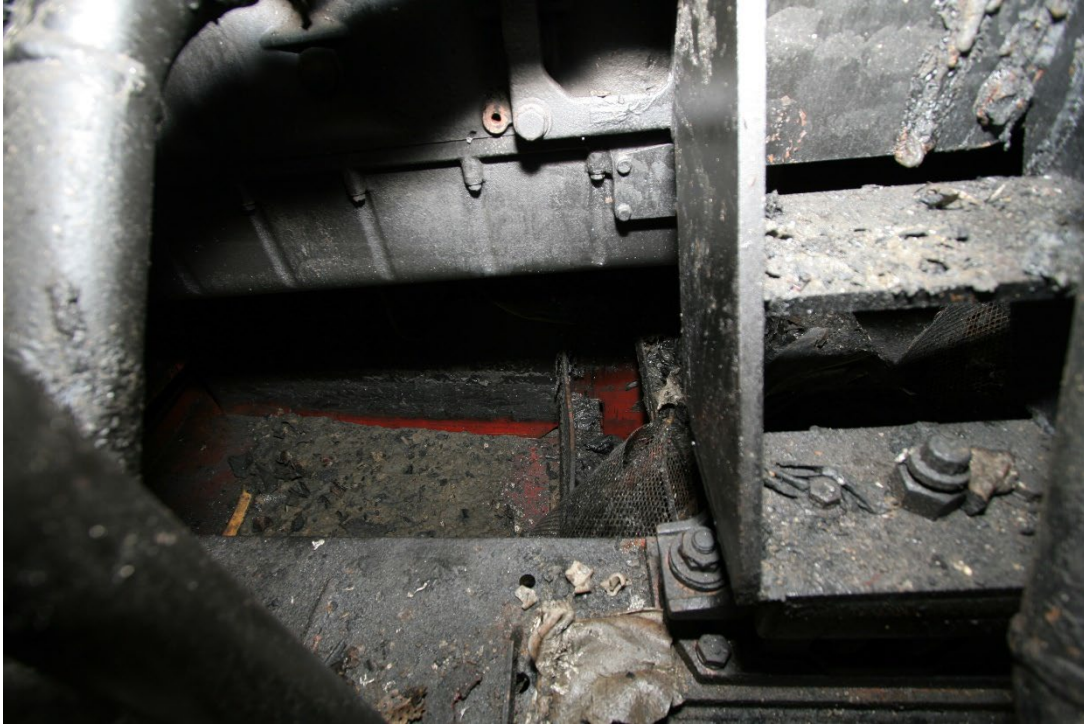
Figure 20. Bilge area below port main engine with some charring on the red paint.
