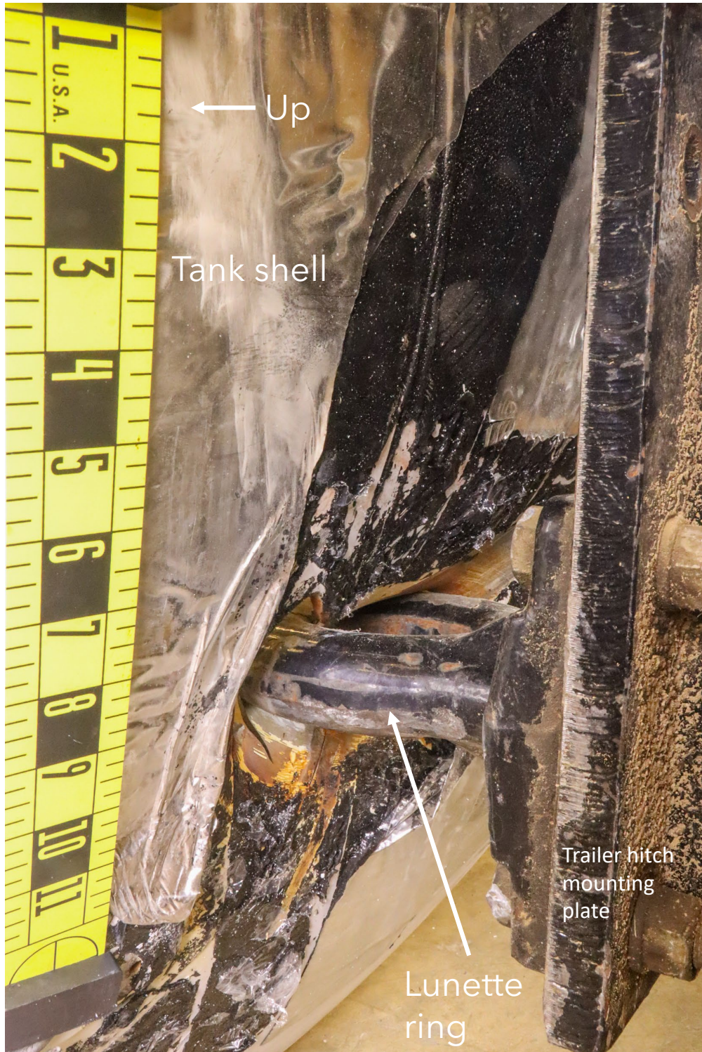
Figure 12. View of the perforation in the exterior side of the front head shell piece A with the trail hitch lunette ring placed close to the perforation.
