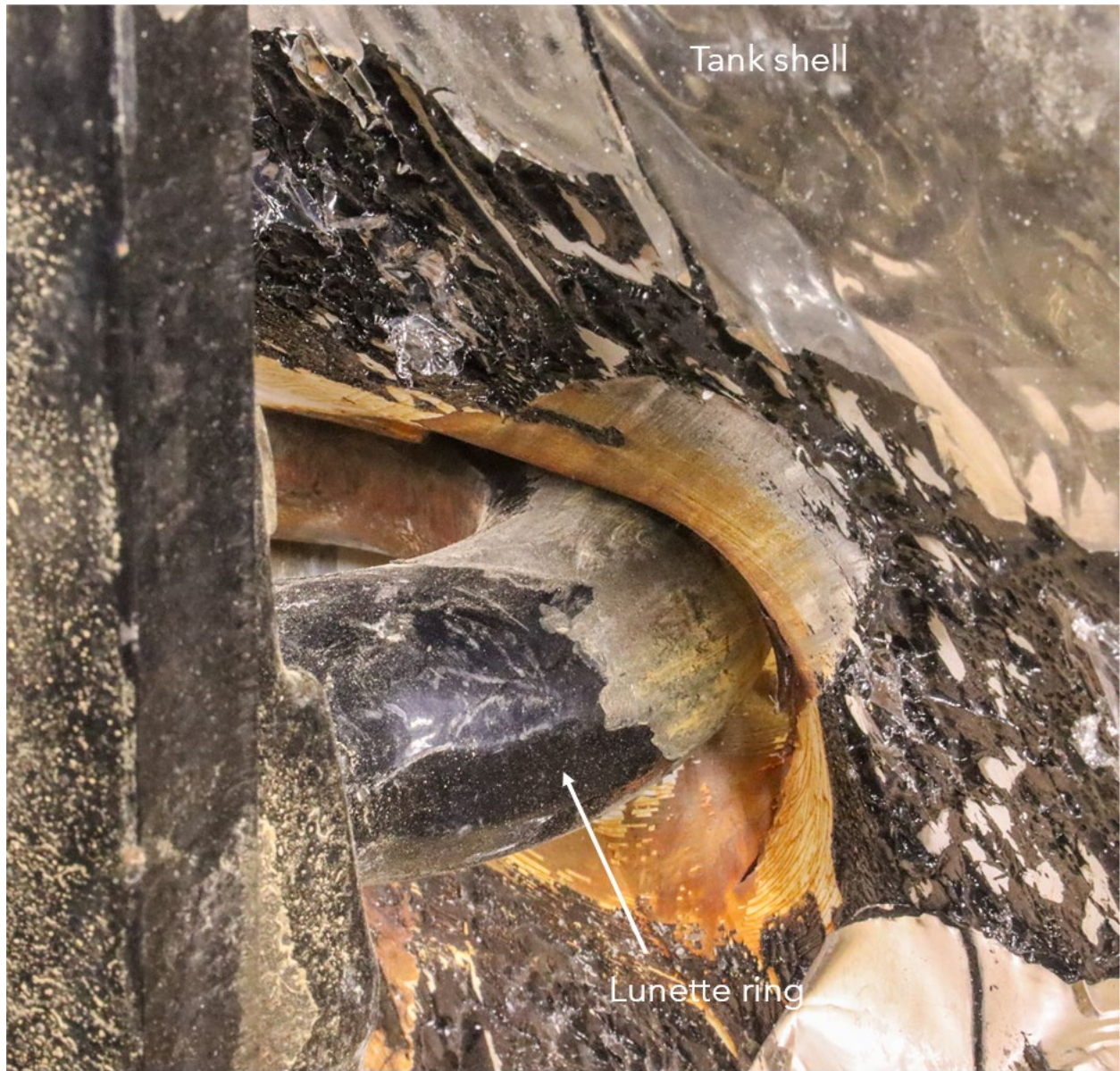
Figure 14. Closer view of the perforation in the exterior side of the front head shell piece with the trail hitch lunette ring placed close to the perforation.
