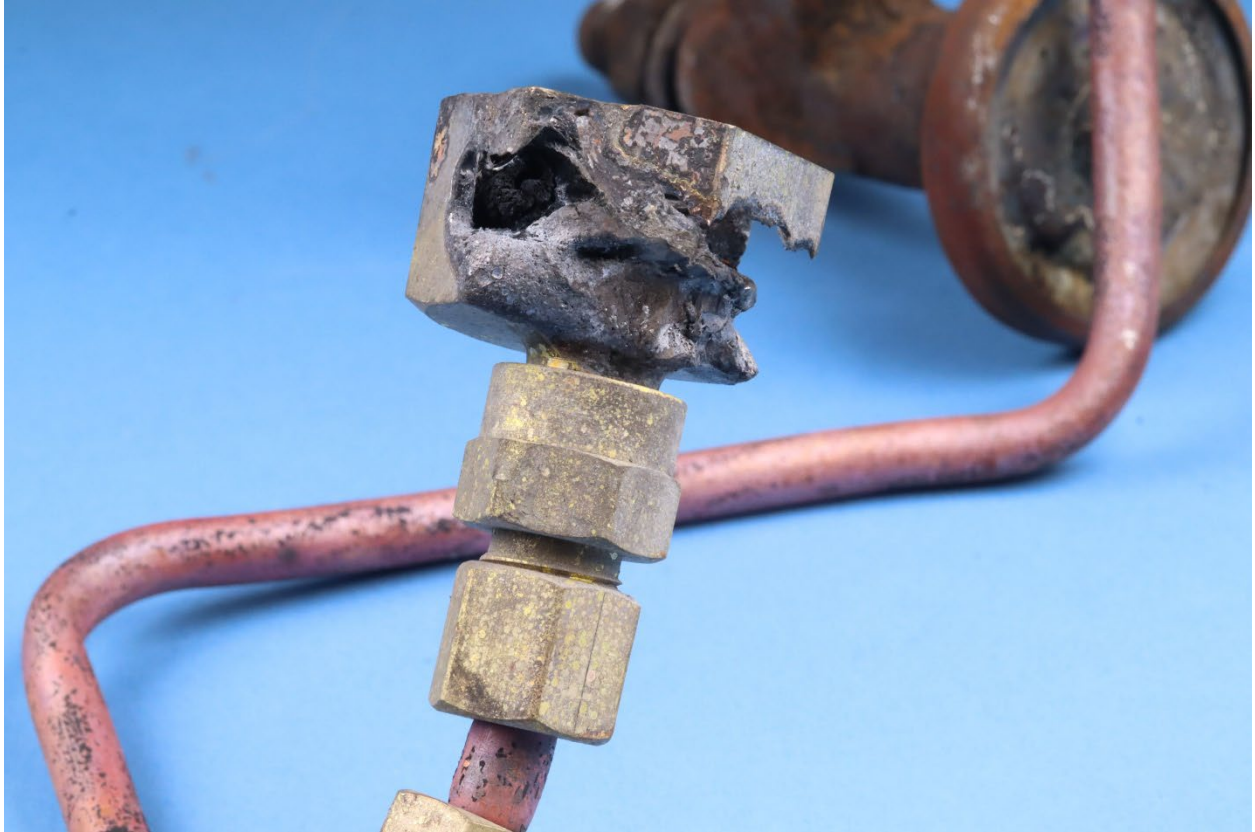
Figure 11. Branch line with damaged fitting on the end.
