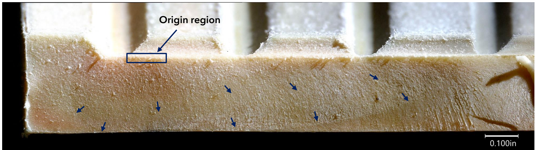
Figure 13. Upper image: Longitudinal fracture from top of tower to base of tower. Lower image: Detailed image of slow crack growth region with blue arrows indicating the local direction of crack propagation.
