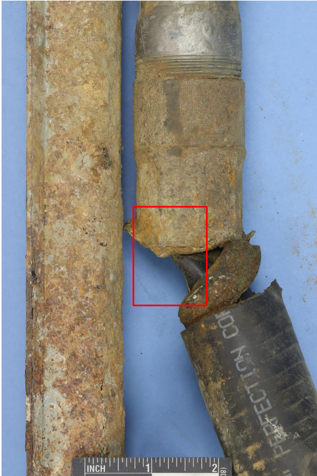
Figure A1. Closer view of flexible riser downstream end showing separation of coiled winding and deformation to end fitting.
