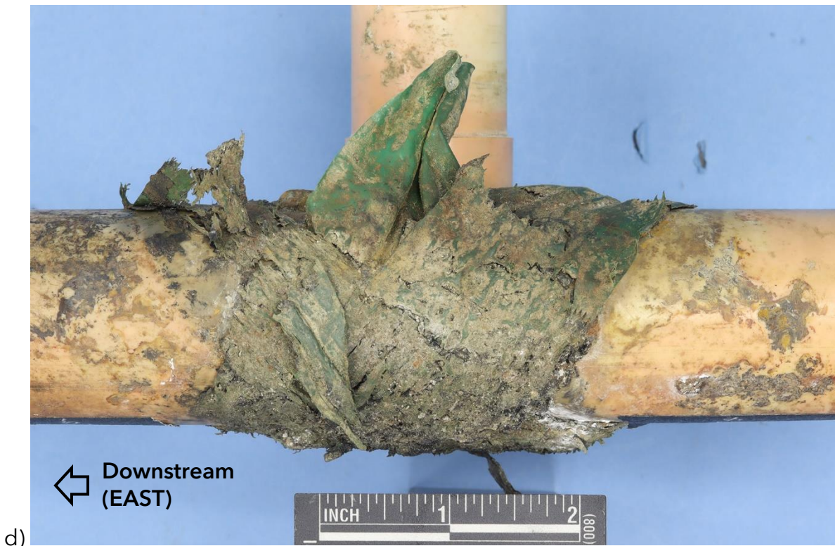
Figure 6 (cont.). c) image showing the appearance of the green tape on the top west side of the tower; and d) image showing the appearance of the tape on the underside of the tower.
