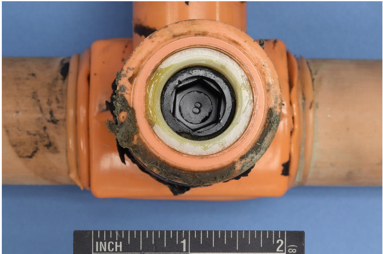
Figure 25. Sister tee from 77 S. 2 nd Ave after removal of the cap showing grease on the insert and cutter.
