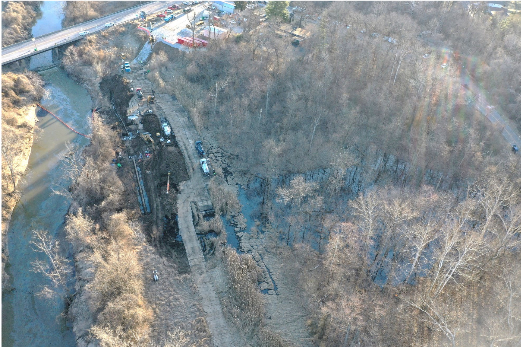
Figure 1. Leak source area, Cahokia Creek, Edwardsville, Illinois. March 13, 2022, 8:09 a.m.
