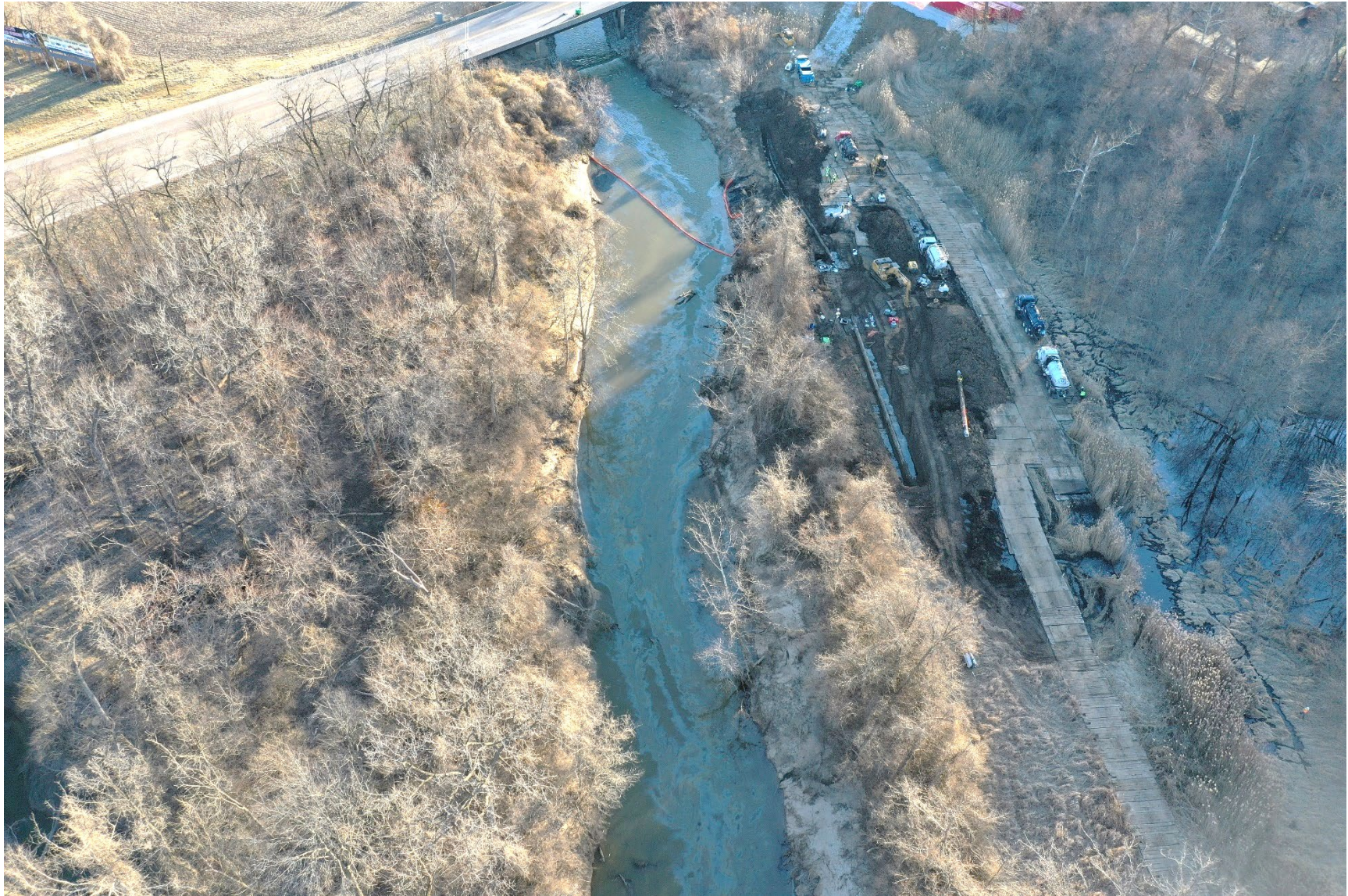
Figure 2. Division 1 leak site, Cahokia Creek, Edwardsville, Illinois. March 13, 2022, 8:11 a.m.
