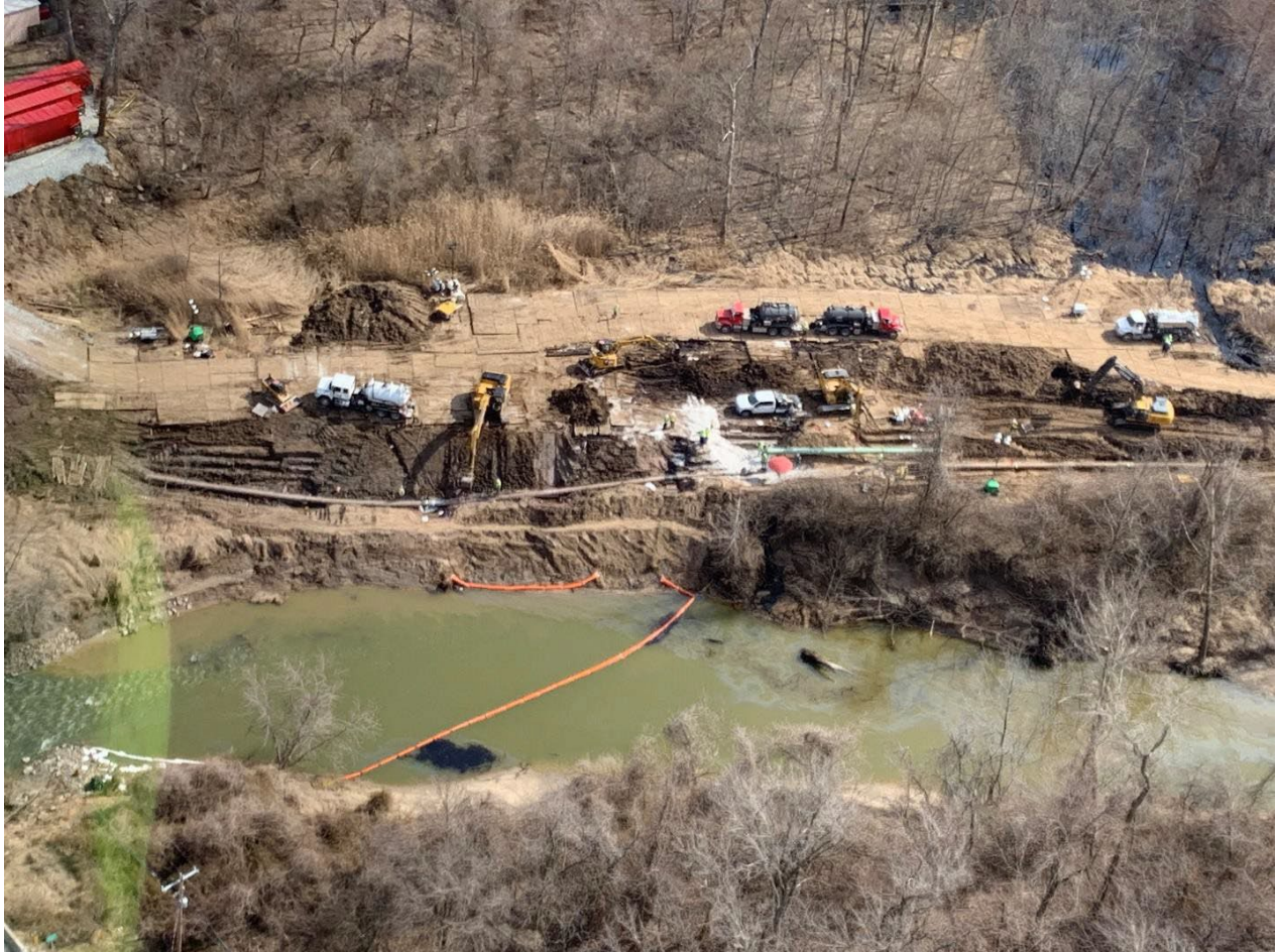
Figure 1.2: Aerial Image of Failure Location
