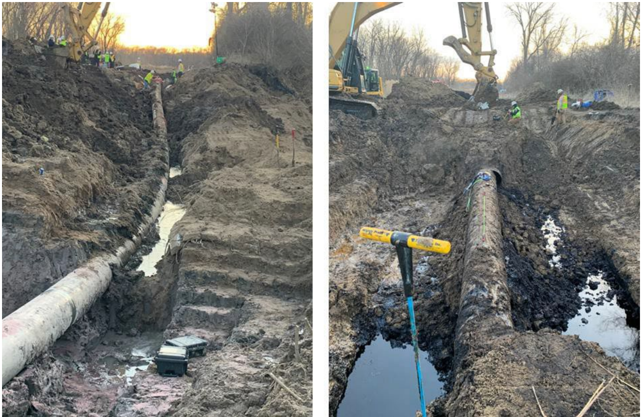
Figure 1.1: Failed Girth Weld During Excavation
