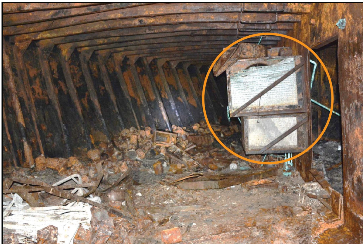
Figure 11. The two compressors (circled in orange) in the dry stores room. The one for the freezer is on top; the one for the chiller is on the bottom . (Background source: ATF)
