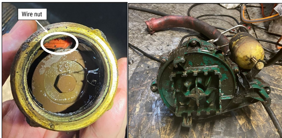
Figure 8. Spring-loaded check valve shown with lodged wire nut ( left ) and associated cofferdam bilge pump with inlet shown with strainer removed ( right ). (Source: Coast Guard)
