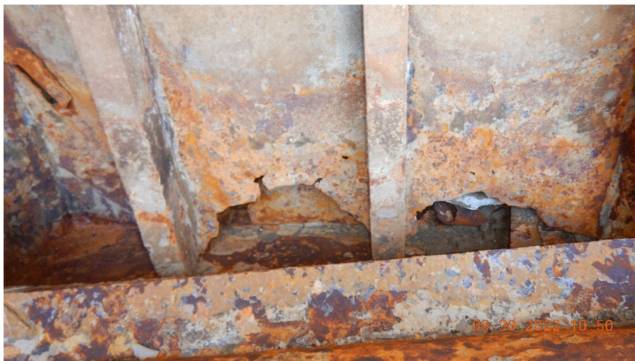
Figure 7. The bottom of the centerline longitudinal bulkhead between the no. 1S and no. 1P compartments of the port barge showing metal loss and corrosion holes. (Source: K. Smith Marine Surveying)
