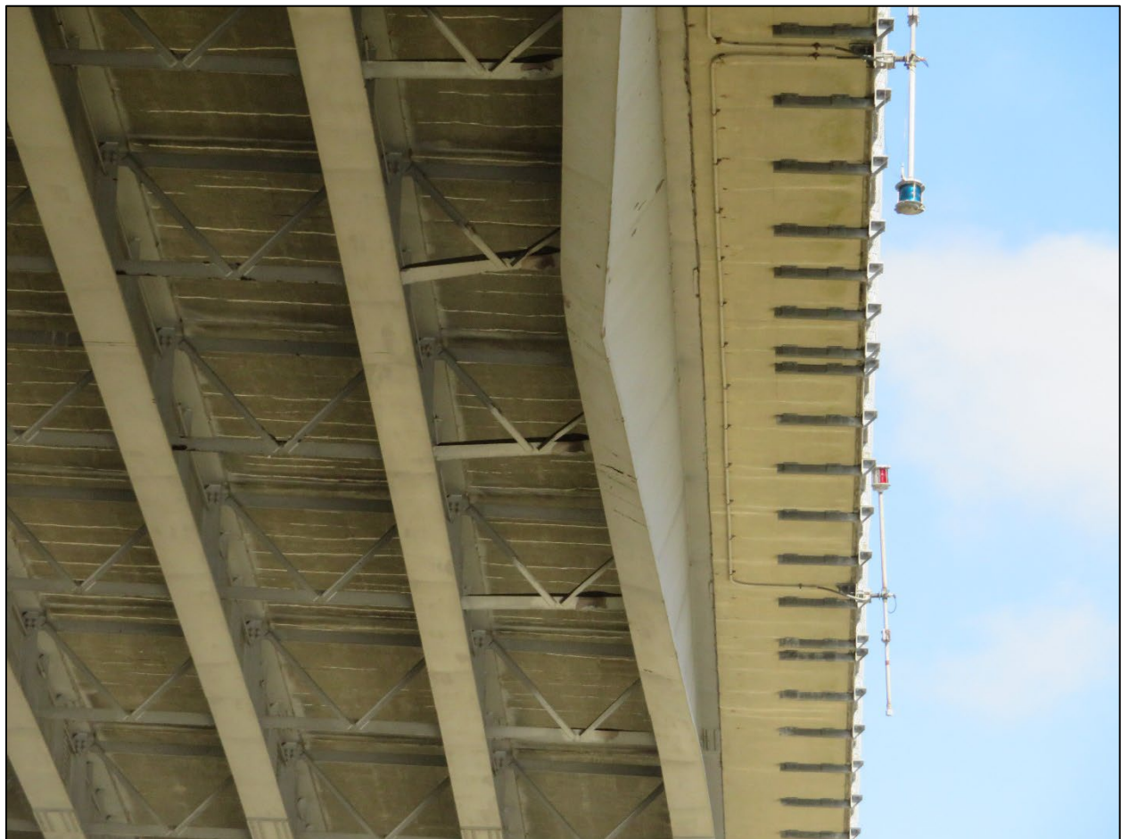
Figure 5. Eastbound span of the Houma Twin Span Bridge showing damaged stringer.
