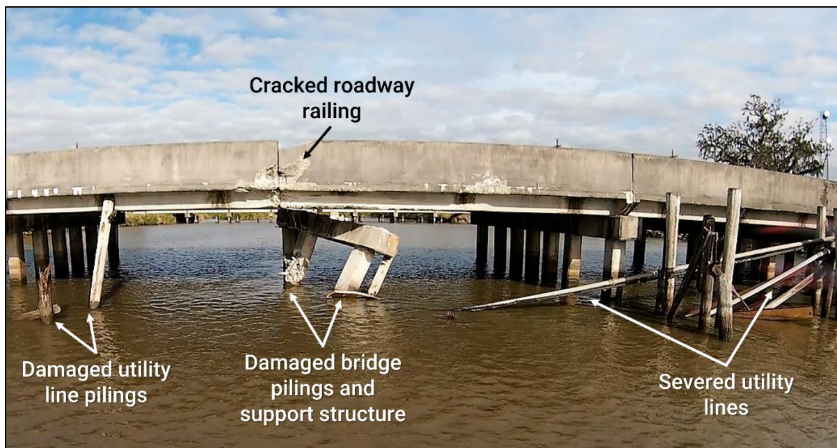
Figure 5. Route 182 bridge damage. (Background Source: Coast Guard Cajun Drone Photography, Jim Pierce Jr. )
