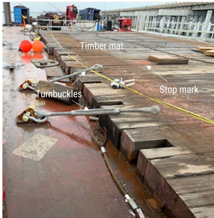
Figure 6. Location of turnbuckles near timber mat and stop mark painted orange on the mat. (Background source: US Coast Guard)
