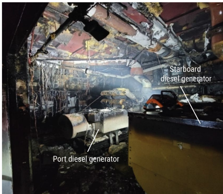
Figure 6. Looking forward in the fire-damaged generator space. The electrical panel foundation where hot work occurred before the fire is in the background, behind the port diesel generator. (Background source: New Orleans Steamboat Company)
