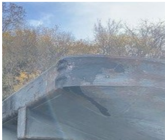
Figure 7. Postcasualty photo of the minor damage to the port bow rake of barge STC 3020 . (Source: Coast Guard)
