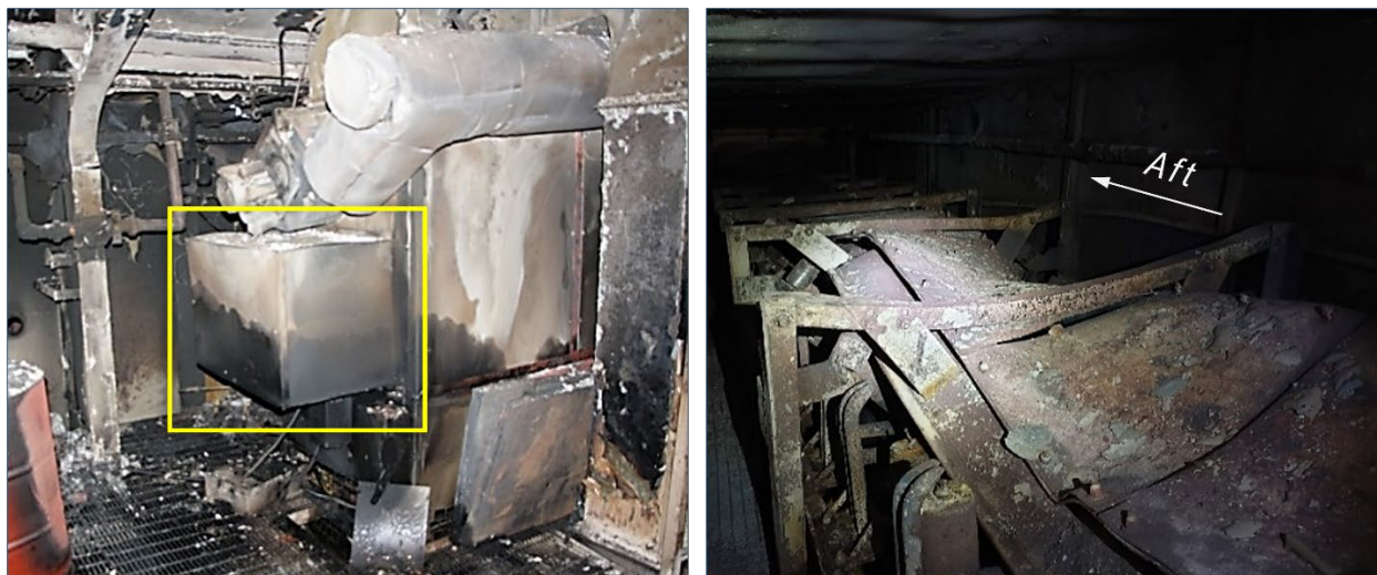
Figure 5. Furnace with burner enclosure outlined ( left ), and fire-damaged conveyor belt within the conveyor belt trunk above the furnace ( right ). (Source: Coast Guard)
