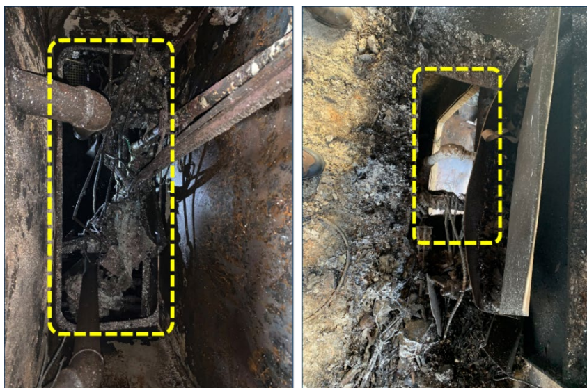
Figure 6. Damaged pipe/hose tunnel, as identified by yellow rectangles, looking up from the engine room ( left ) and down onto the deck winch-control console location ( right ).
