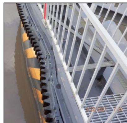
Figure 5. Damaged steel plating and rack on gate.
