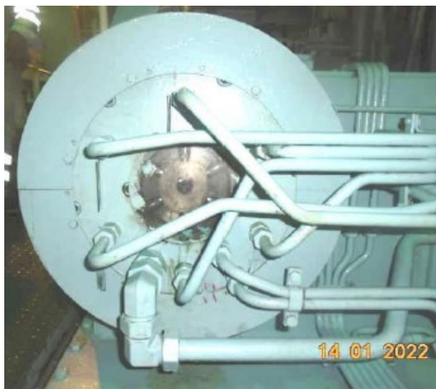
Figure 7. The main engine's starting air distributor containing the no. 6 starting air actuator valve. (Source: Thome Ship Management)
