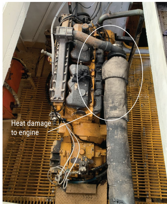
Figure 3. Port main propulsion engine damage on the Desperado after the fire.
