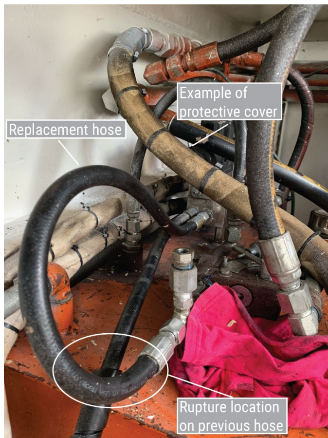
Figure 5. The replacement hydraulic hose, with the location of the rupture on the previous hose circled.
