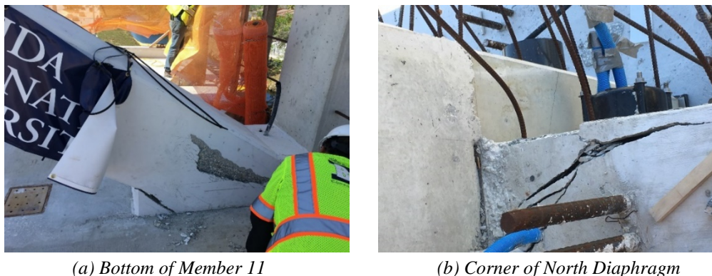
Figure 2. Cracks at north end of Main Span (Node 11/12) on March 14, 2018, showing examples of cracking discovered in the Main Span prior to the collapse. 2
