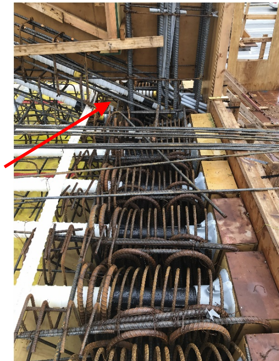
Figure 19. July 25, 2017: Forms, reinforcement, and PT at Type I Diaphragm and Truss, location of construction joint indicated with red arrow. 78
