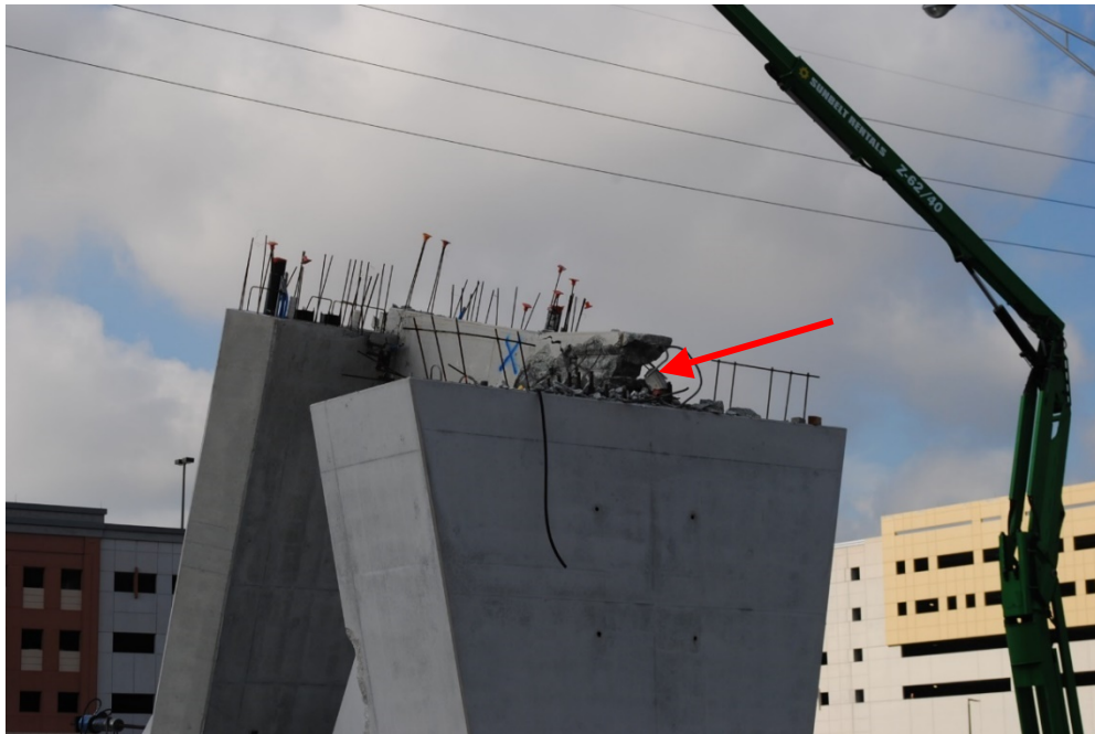
Figure 59. Fractured surface at base of Member 12 (indicated with red arrow).
