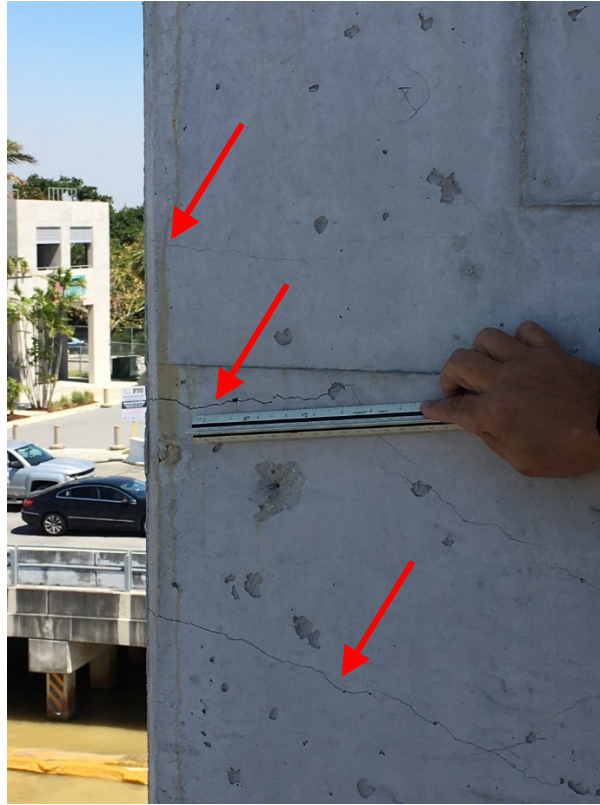
Figure 51. Flexural cracks on north face of vertical Member 12 (indicated with red arrows). 192
