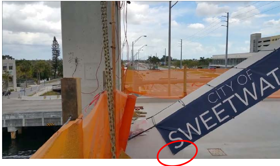
Figure 40. Node 11/12 after erection and before destressing of Diagonals 2 and 11 (location of repaired crack indicated with red circle). 129
