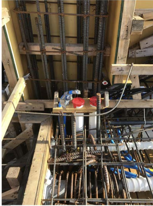
Figure 30. Deck and Web forms and reinforcement prior to pour of Deck concrete (Member 12). 101
