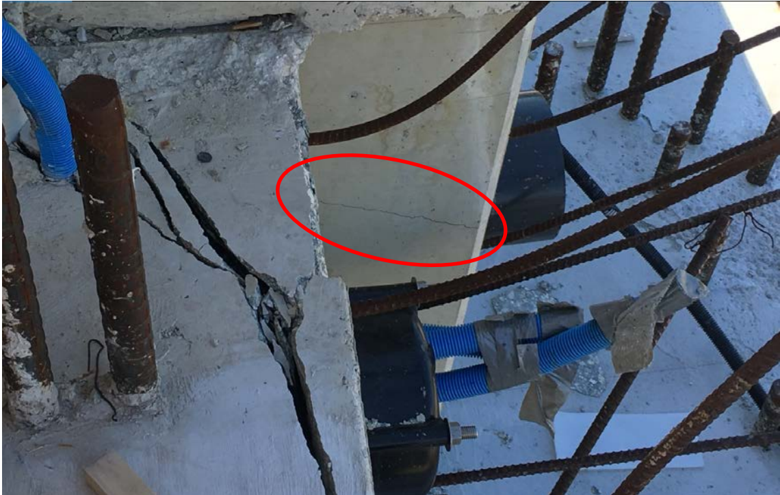
Figure 58. Diagonal crack in vertical Member 12 (indicated with red circle). 201
