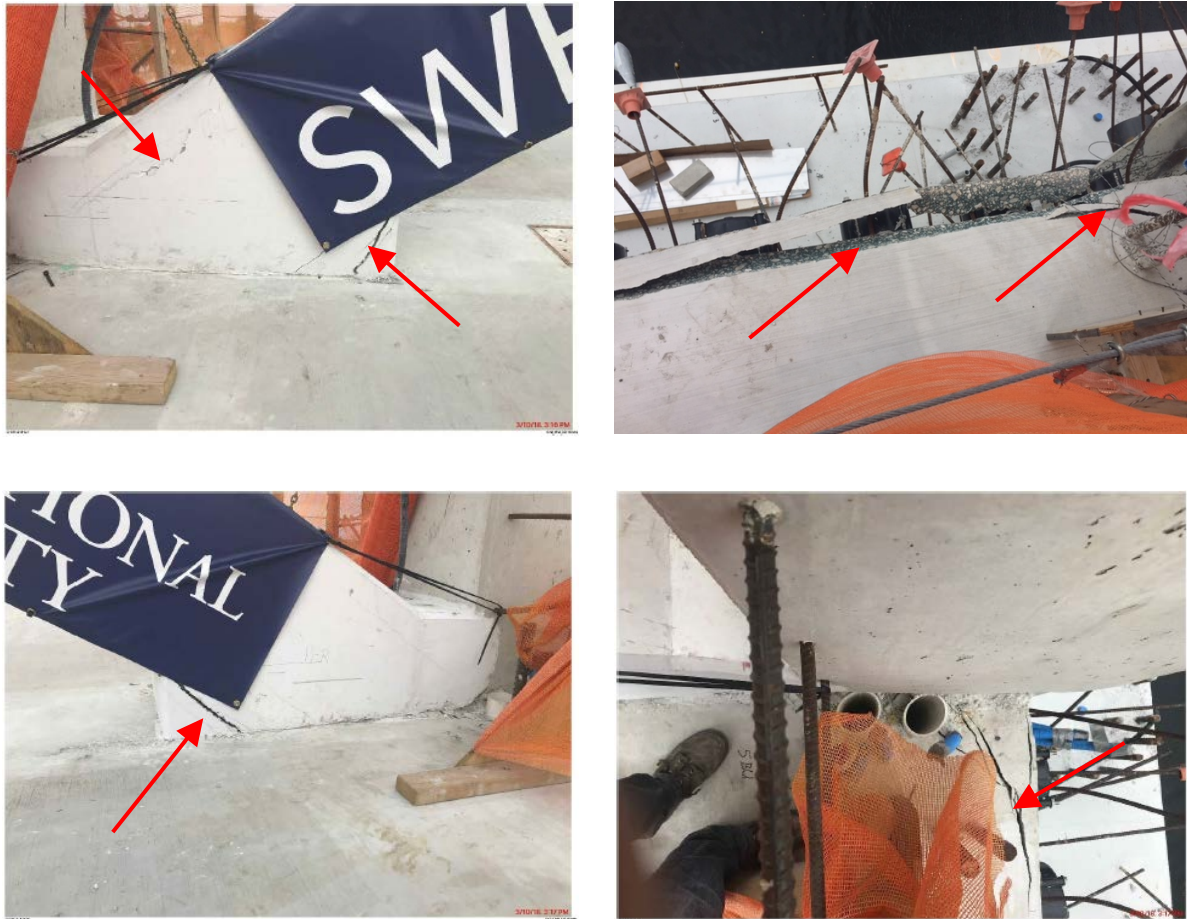
Figure 41. Cracks observed after initiation of destressing on March 10, 2018, at north end of Main Span (indicated with red arrows). 134
