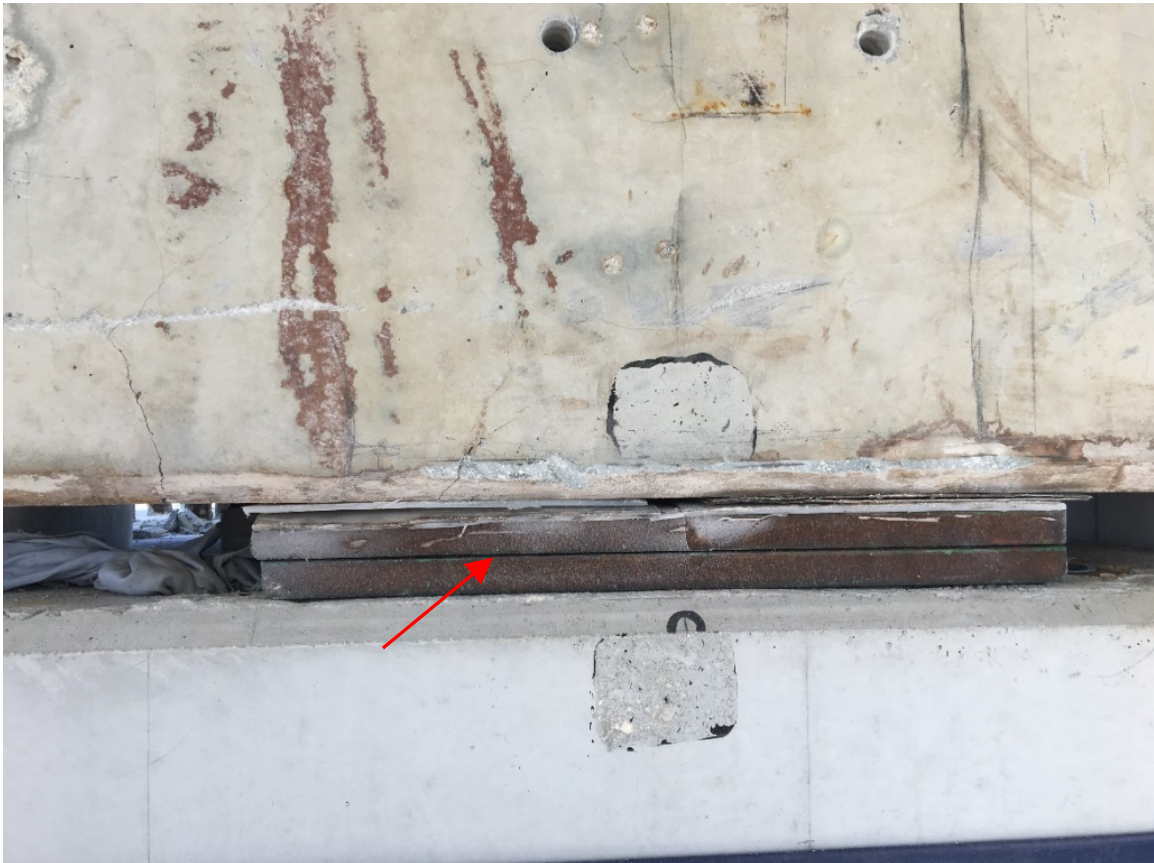
Figure 42. Steel shims under vertical Member 12 on March 13, 2018 (indicated with red arrow). 151
