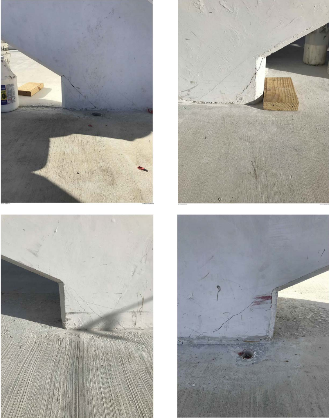
Figure 37. Cracks after removal of forms and shoring on February 26, 2018. 122
