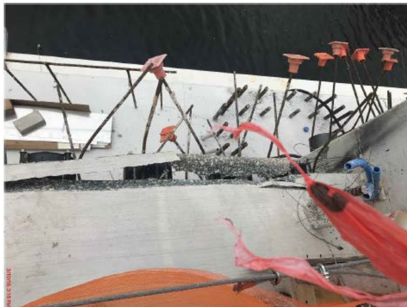
Figure 52. Spalling along top corner of Type II Diaphragm. 193
