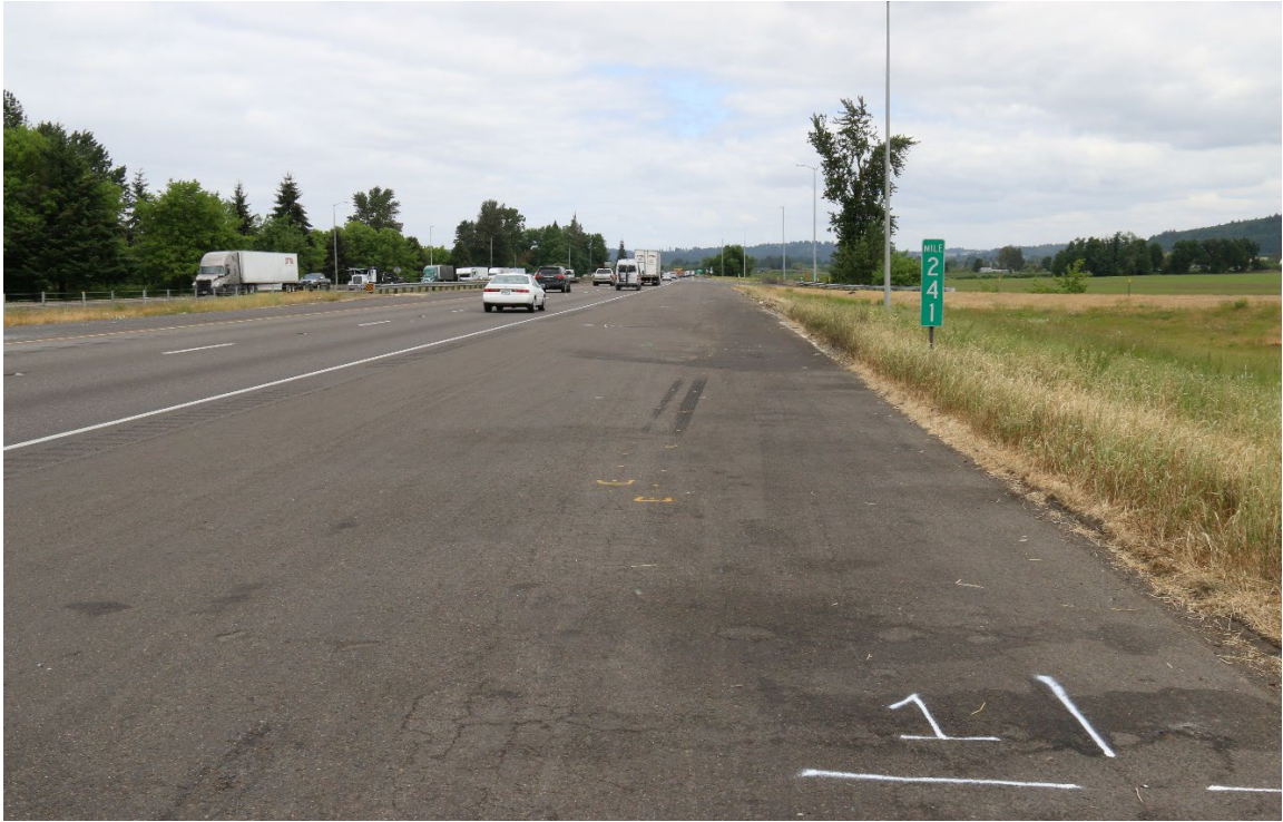
Figure 2: Photo of the shoulder looking North at the Santiam Rest Area on I-5.
