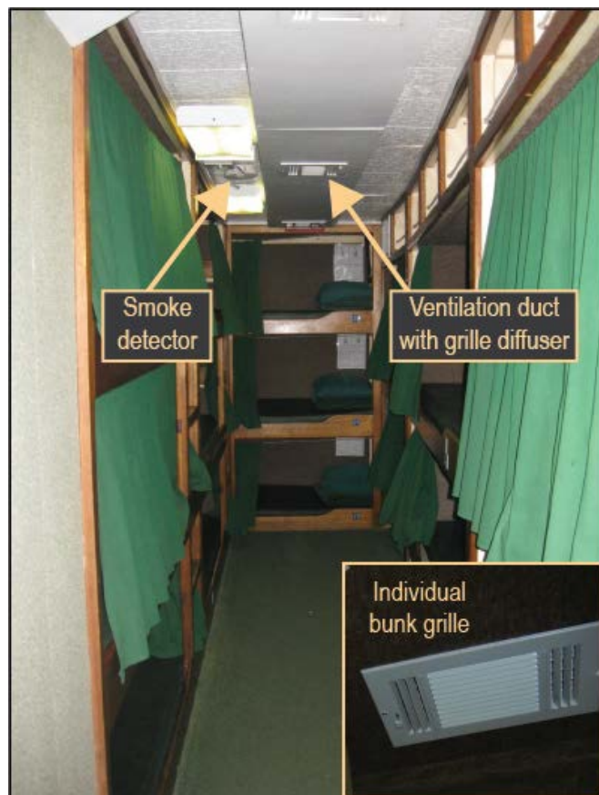
Figure 16. Port side of the Conception's bunkroom looking aft, with inset of grille/diffuser. (Source: M. Ryan; Inset: S. Landis)
