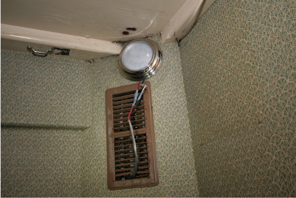
Figure 23. Power cable for lighting routed through ventilation grille in the Vision's bunkroom.
