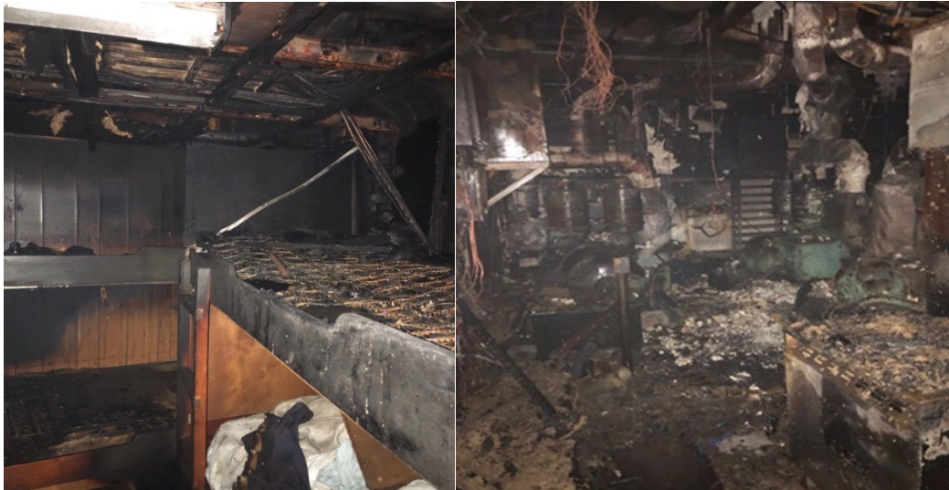
Fire damage to living quarters (left) and generator room (right). (Source: Coast Guard)
