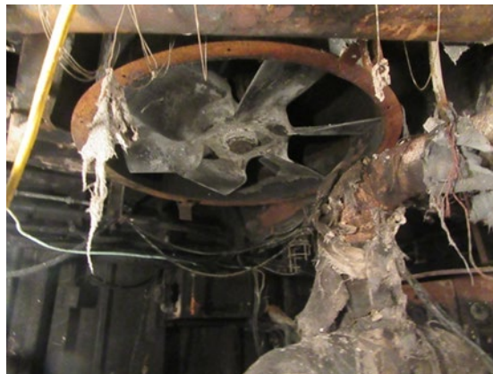
Starboard exhaust trunk fan (post-fire) located above the number one generator. (Source: Coast Guard)
