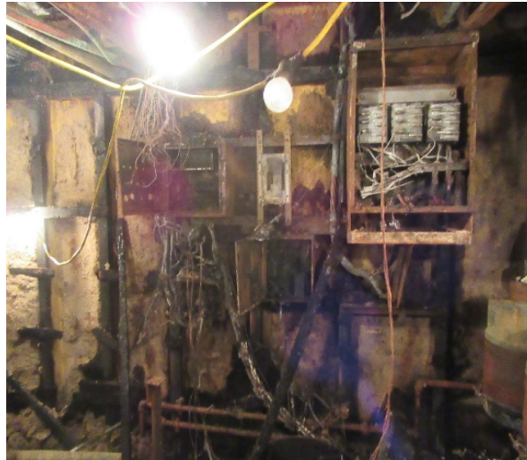
Forward bulkhead of the generator room where the source of the fire was identified by the LaFourche Parish Fire District (Source: Coast Guard)
