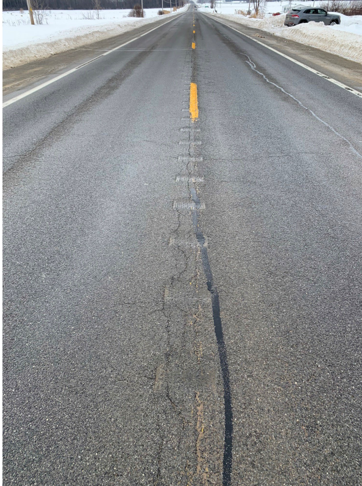
Figure 3 - View of centerline rumble strips along State Route 37 in the vicinity of the crash
