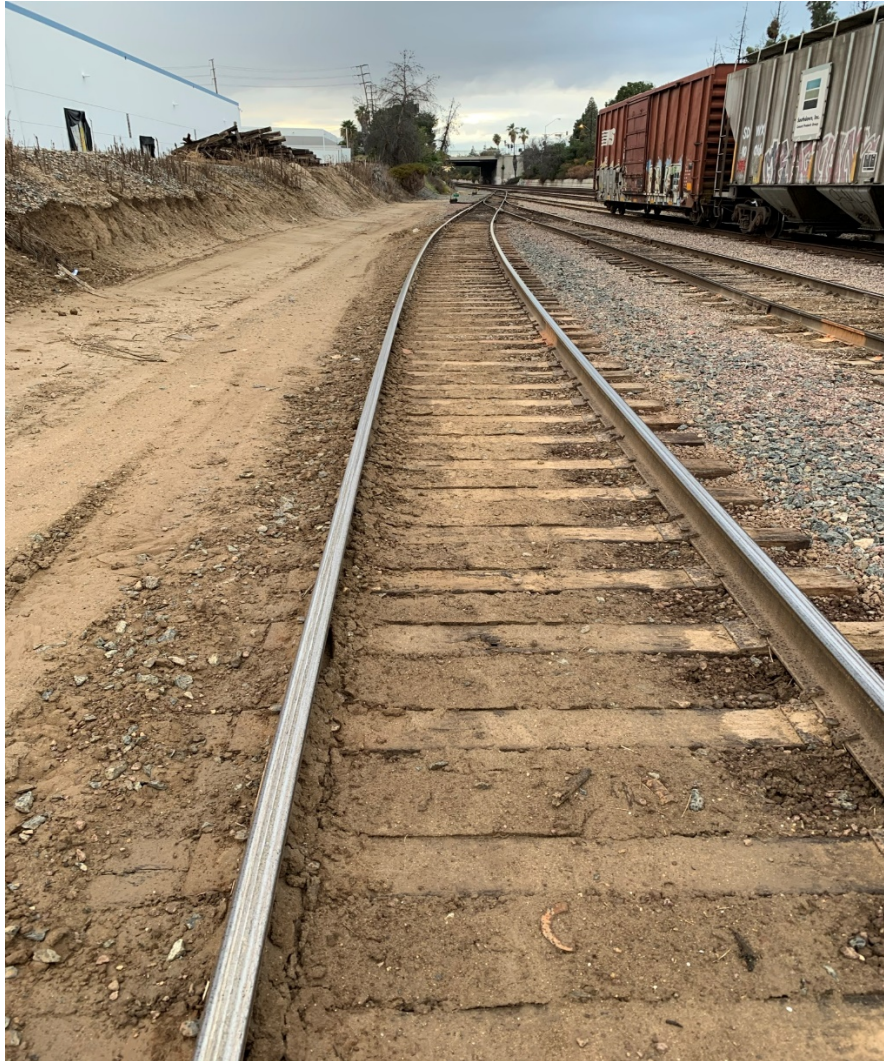
Figure 7: Photograph taken looking west at the west end of the railyard. Faded paint indicating a clearance point is located on the base and web of the rail of several yard tracks.
