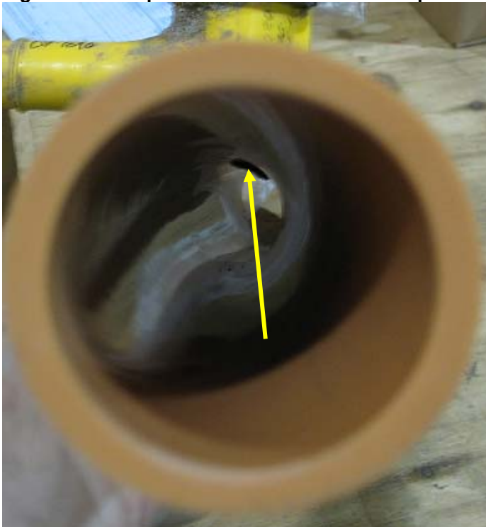
Figure C4: Sample 07-1090 Interior View of Tap
