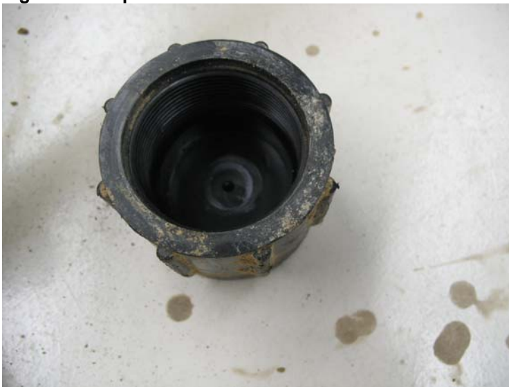
Figure D1: Cap As-Removed
