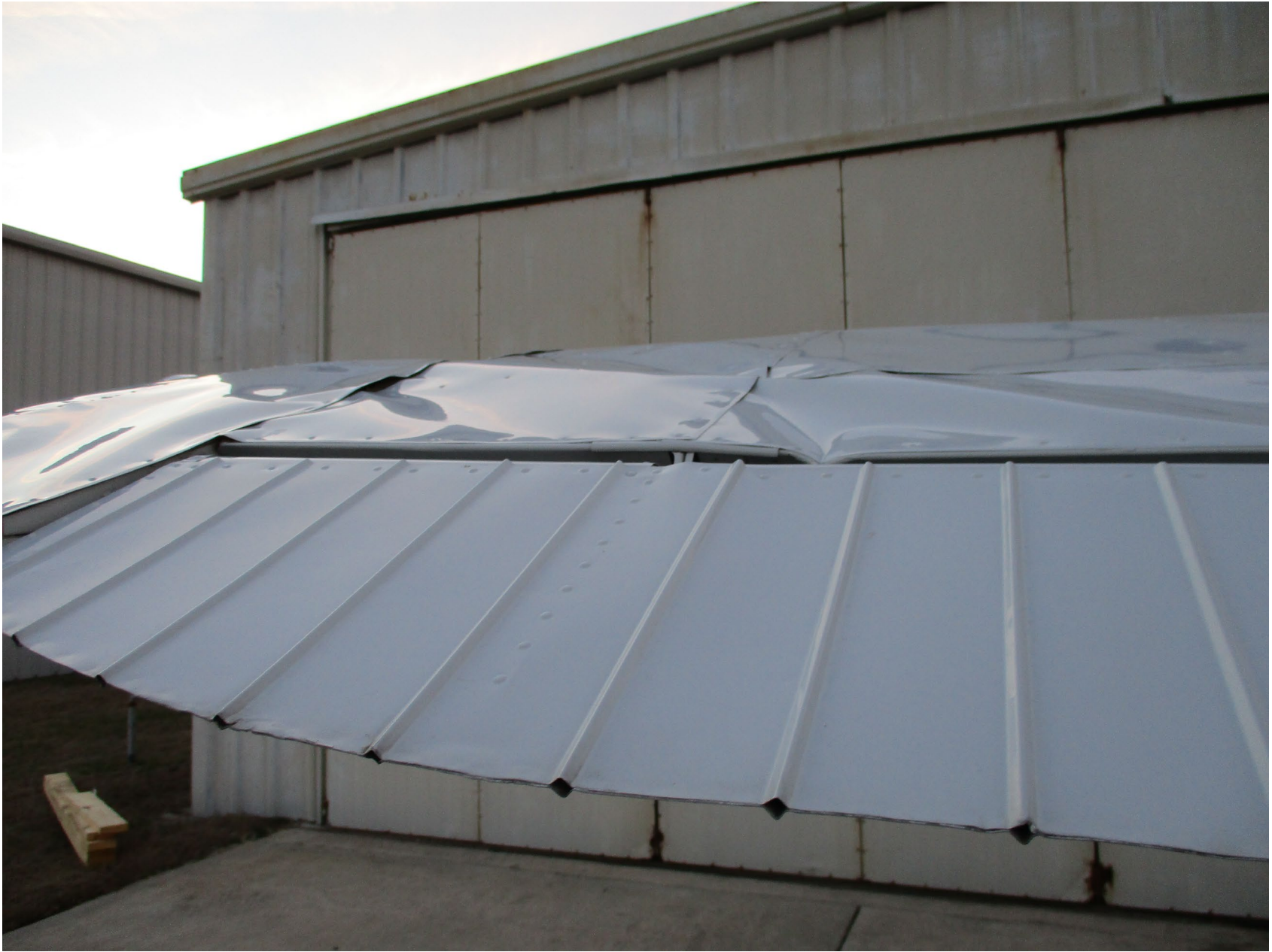
Photo 2 – Close-up view of left damaged wing
