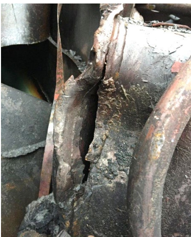
3(e) Impact mark B-end head brace, head brace weld, and fractured head pad.
