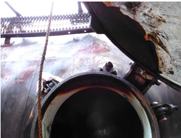
6(c) Manway and burnt gasket and interior cover surface.
