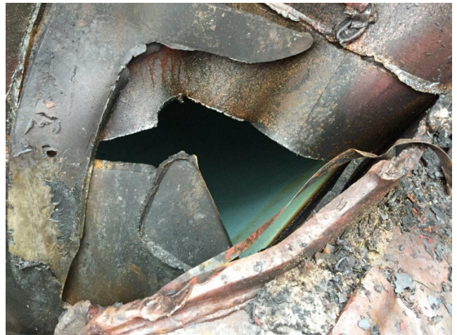
3(d) Fractured B-end head pad and hole in tank.
