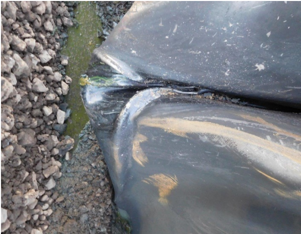
4(c) A-R buckled tank shell, cracked, and releasing material.
