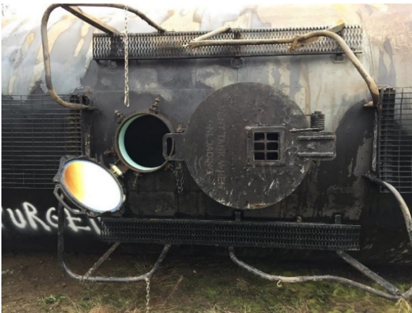
8(c) Top fittings, thermal damage to manway cover.
