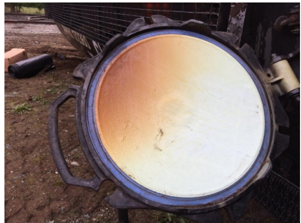
8(d) Manway cover, interior surface thermal damage.
