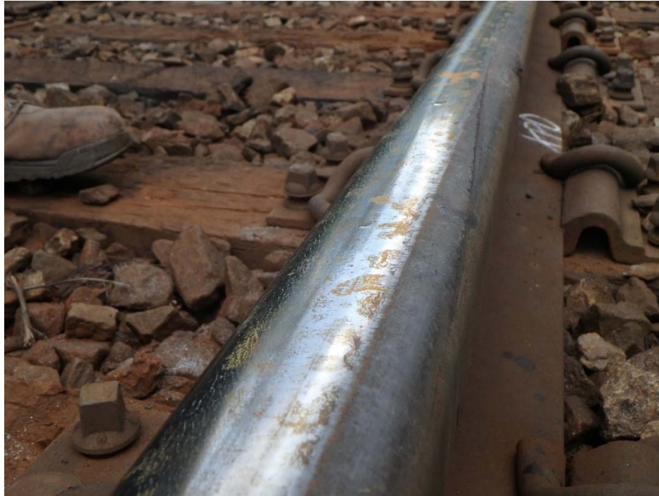
Figure 2. Photo showing wheel flange departure mark across high rail in curve at POD.
