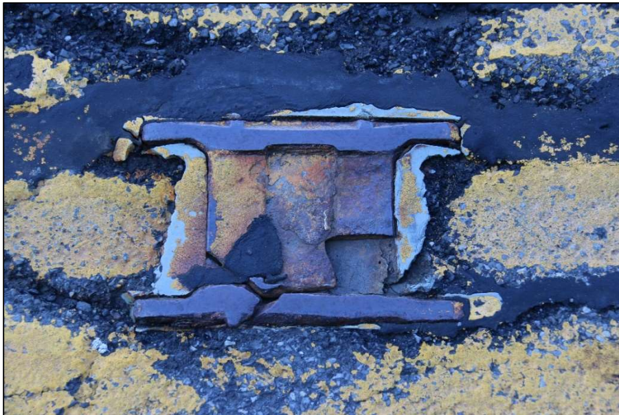
Figure 5: Example of degraded centerline retroreflective raised pavement marker.
