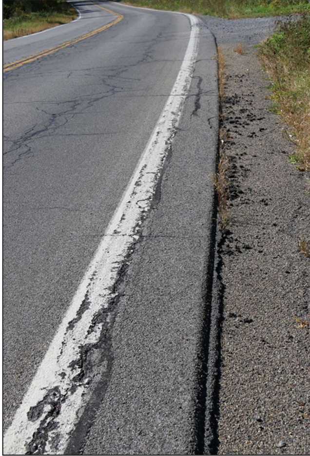
Figure 4: Photograph depicting an example of pavement edge and edge line condition. View is looking southward.
